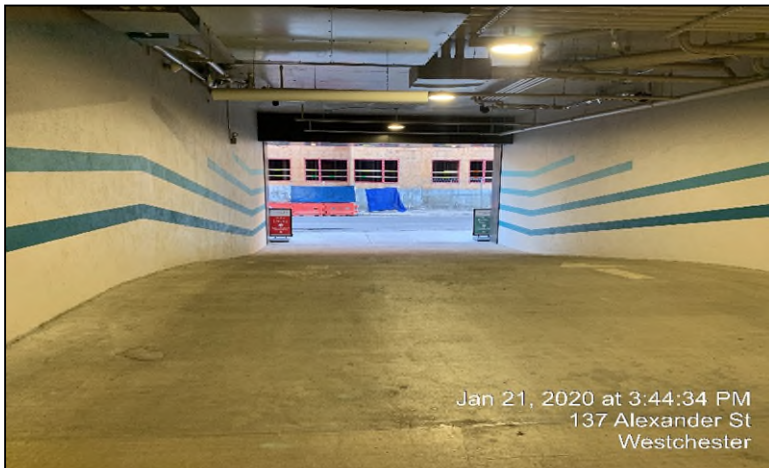
Photograph 15: The parking garage entrance ramp on the northeastern portion of the Site.
