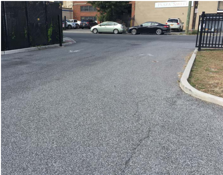
Photograph 1: Onsite asphalt is in good condition with no evidence of penetrations or major cracks (Location OSMW-04, looking southeast to west-northwest).
