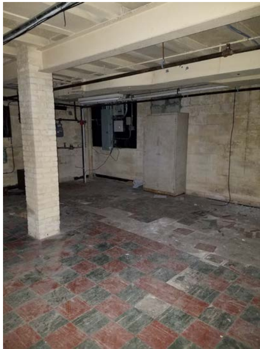
Photograph 5: Some tiles are missing from the floor at 441 Waverly Avenue; however, floor is in acceptable condition. No evidence of cracks or penetrations were observed (looking southeast to northwest).
