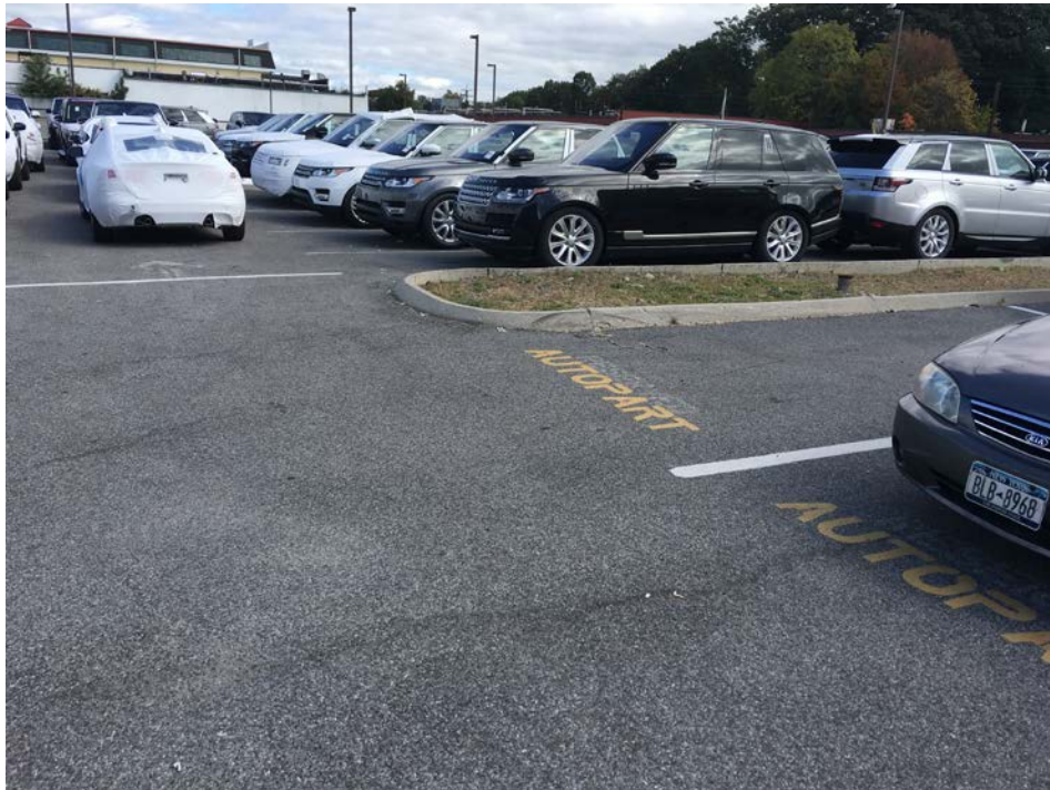
Photograph 4: Curbed areas and asphalt cover system are in good condition with no evidence of erosion or cracks (looking southwest to northeast).
