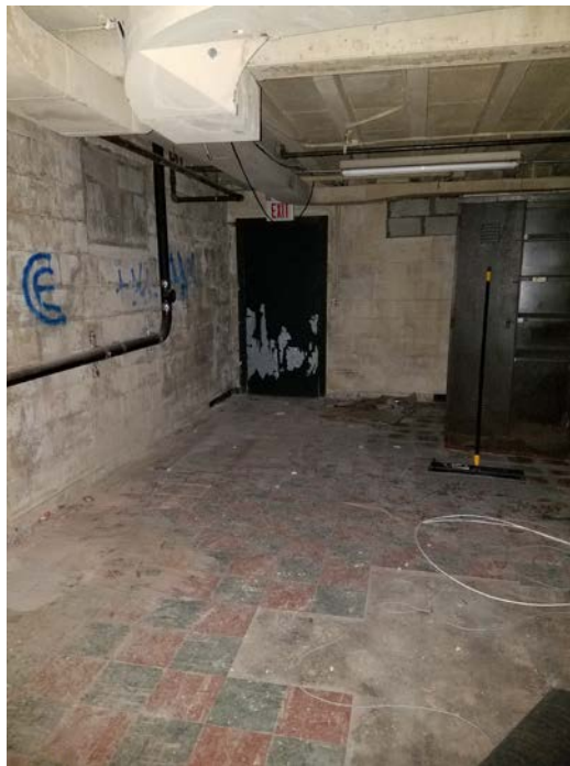
Photograph 6: Some tiles are missing from the floor at 441 Waverly Avenue; however, floor is in acceptable condition. No evidence of cracks or penetrations were observed (looking north).
