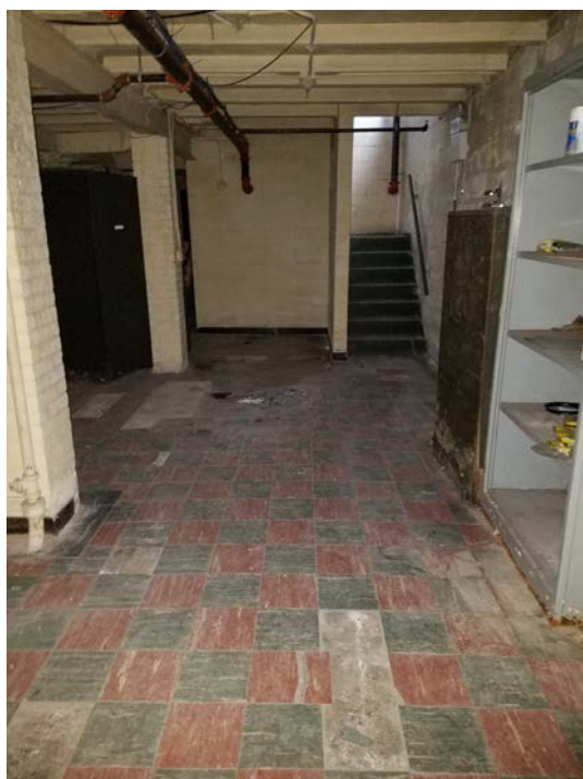
Photograph 7: Some tiles are missing from the floor at 441 Waverly Avenue; however, floor is still in acceptable condition. No evidence of cracks or penetrations were observed (looking northwest to southeast).
