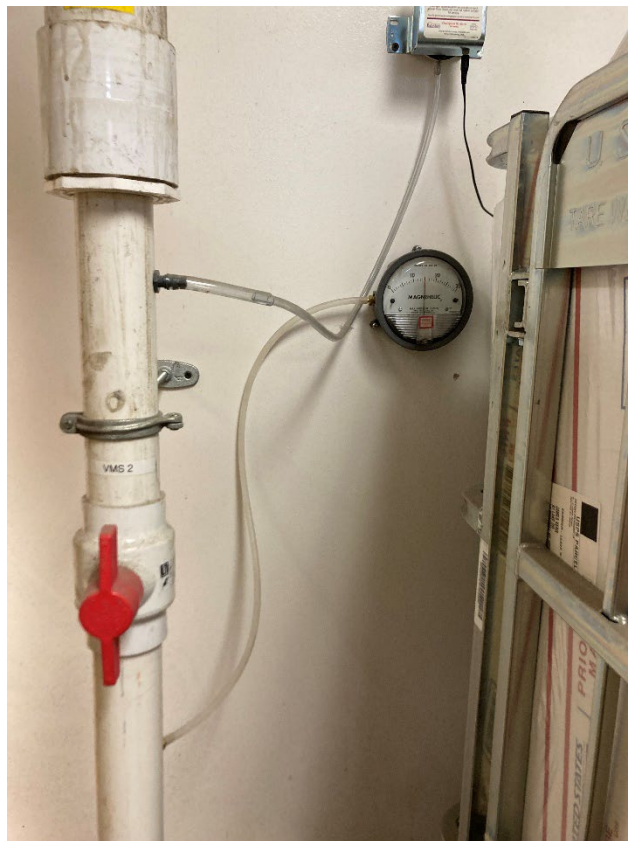
Photograph 16: [5/13/22] Vacuum Reading at extraction point EP-2 inside post office
