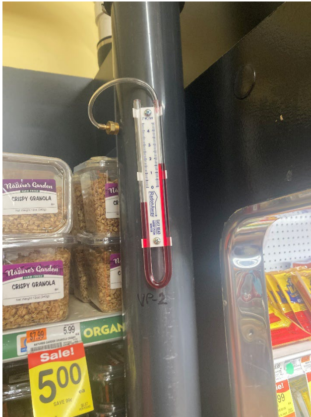
Photograph 8: [5/13/22] Vacuum Reading at extraction point VMP-2
