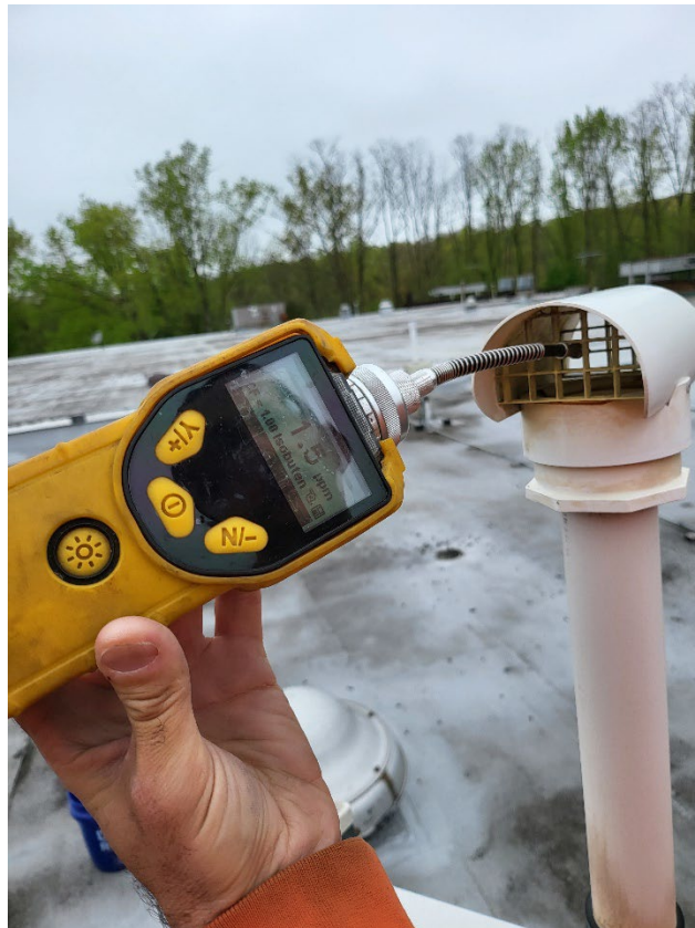
Photograph 18: [5/13/22] Maximum PID reading recorded at discharge stack
