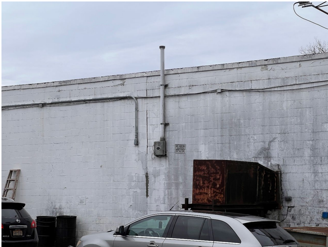
Photograph 11: [5/13/22] View of fan connected to VMP-1 through VMP-3
