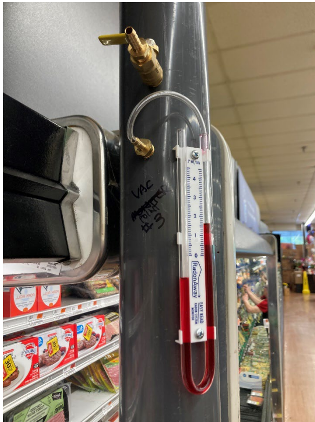
Photograph 10: [5/13/22] Vacuum Reading at extraction point VMP-3
