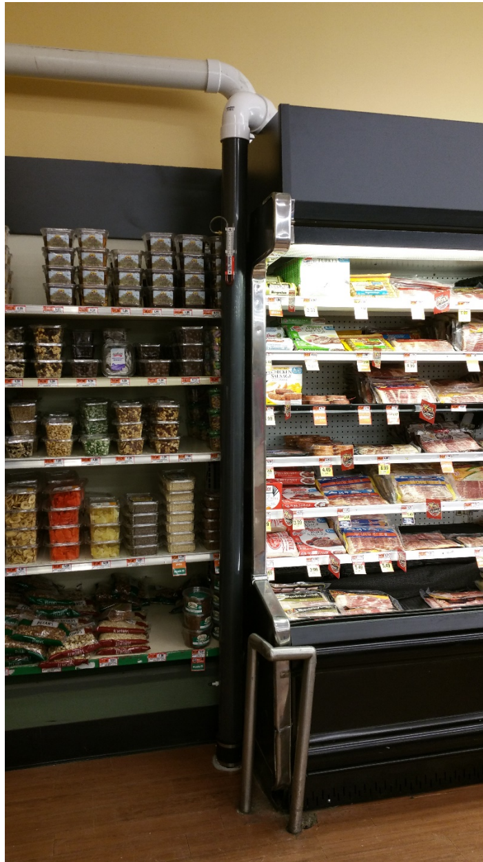
Photo 1 – View of extraction pipe adjacent to sample location 2830-SS-1 by the store room doors.
