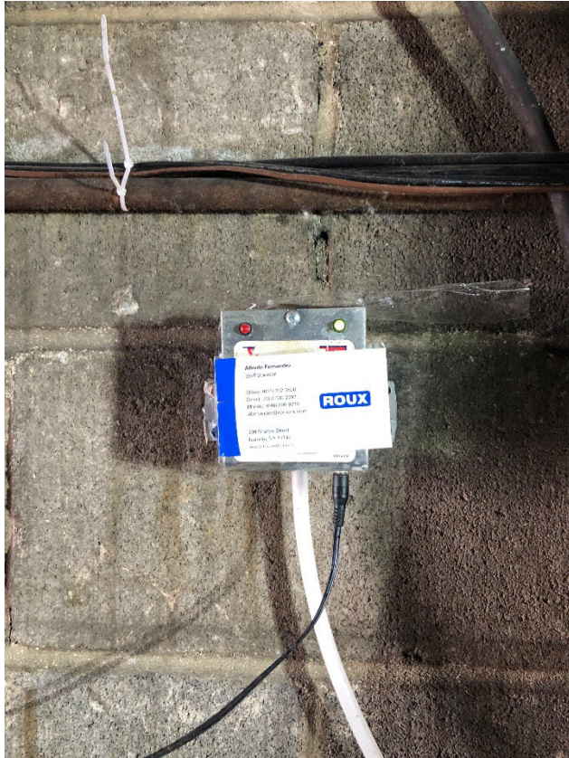
Photograph 24: [2/24/23] Alarm light for EP-1 indicating fan is on
