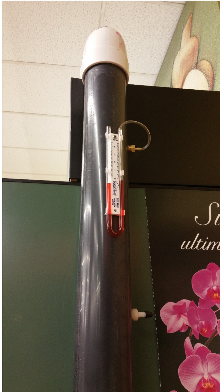
Photo 3 – View of manometer and sampling port on extraction pipe at sample location 2830-SS-3.
