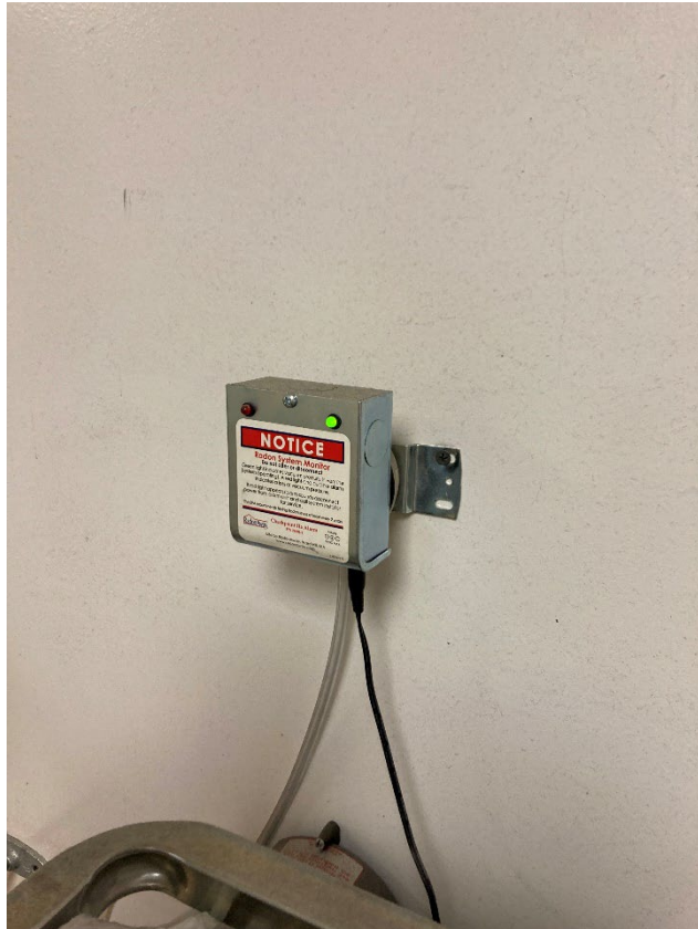
Photograph 19: [5/13/22] Alarm light for EP-2 indicating fan is on
