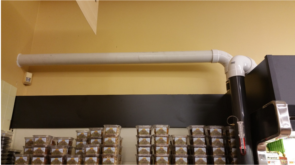
Photo 4 - View of horizontal pipe run penetrating the storeroom wall by sampling location 2830-SS-1.
