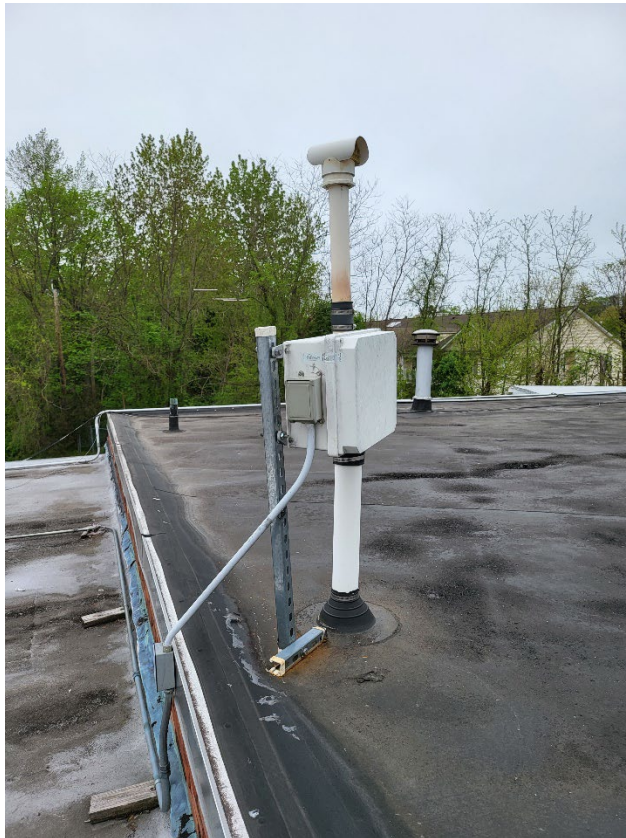
Photograph 20: [5/13/22] RadonAway fan installed at EP-2
