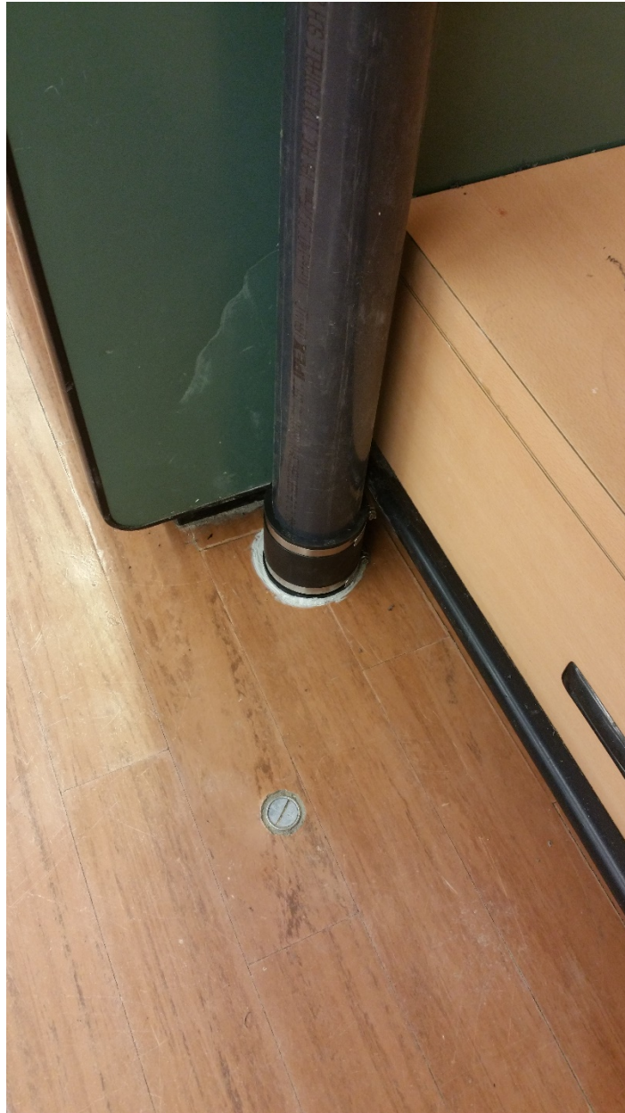
Photo 2 - View of extraction pipe adjacent to sampling location 2830-SS-3 adjacent to the floral department.
