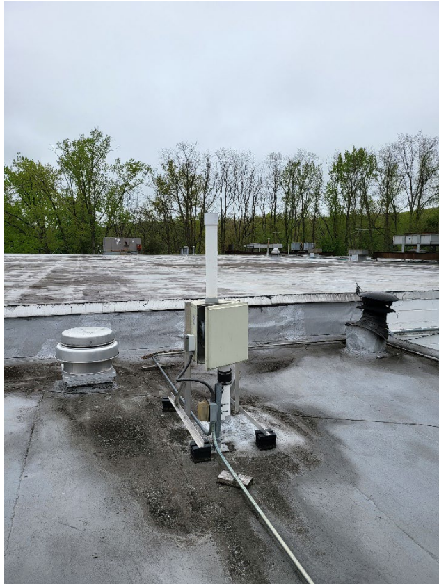
Photograph 17: [5/13/22] Faulty Obar Systems fan installed at EP-1
