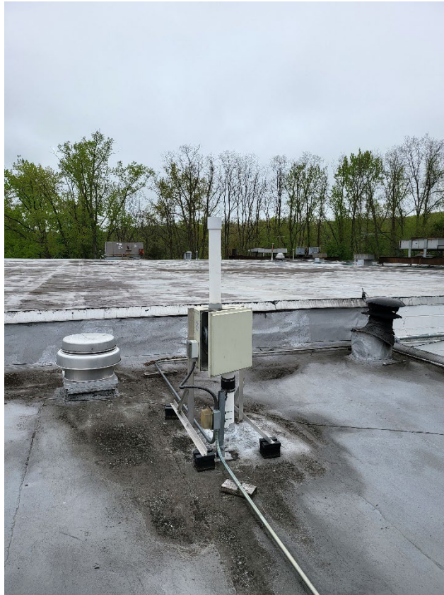
Photograph 17: [5/13/22] Faulty Obar Systems fan installed at EP-1
