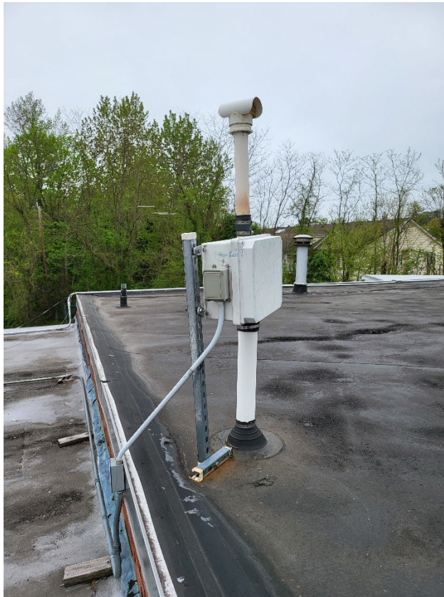
Photograph 20: [5/13/22] RadonAway fan installed at EP-2
