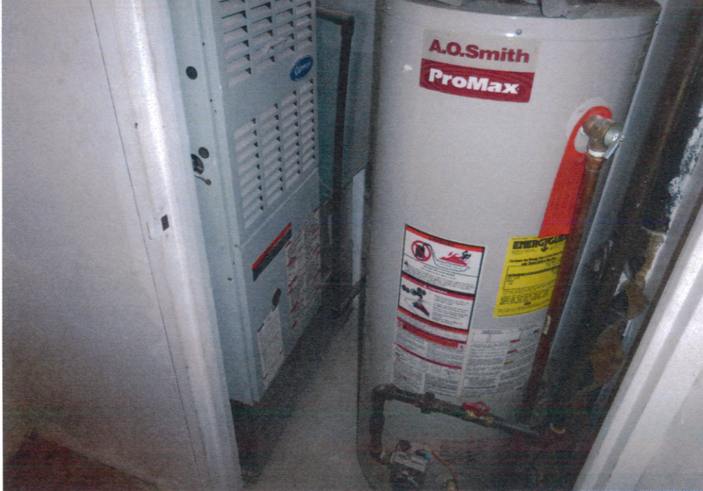
TOWNHOUSE UNIT FURNACE AND HOT WATER TANK
