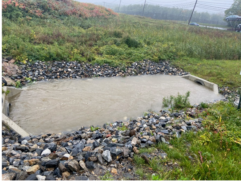
Photo 13 – Outfall 7 during heavy rain event, October 26, 2021
