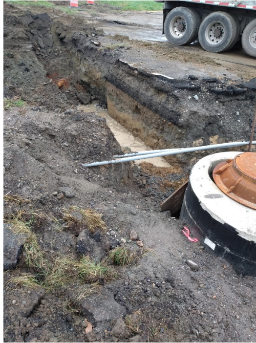
Photo 1 – Water in trench near MH-7024
