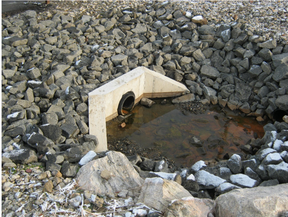
Photo 3 – Steady state flow at MH-7015.1
