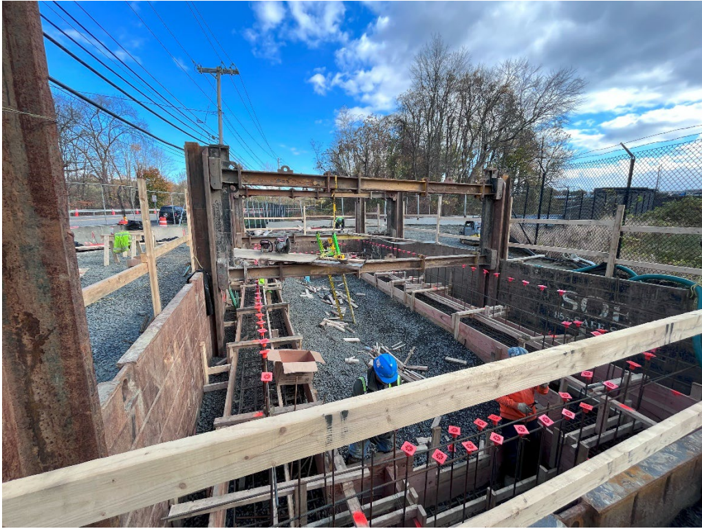
Photo 1 – Progress made as of 11/1/23. The photo shows the forms for the footing and rebar being installed.
