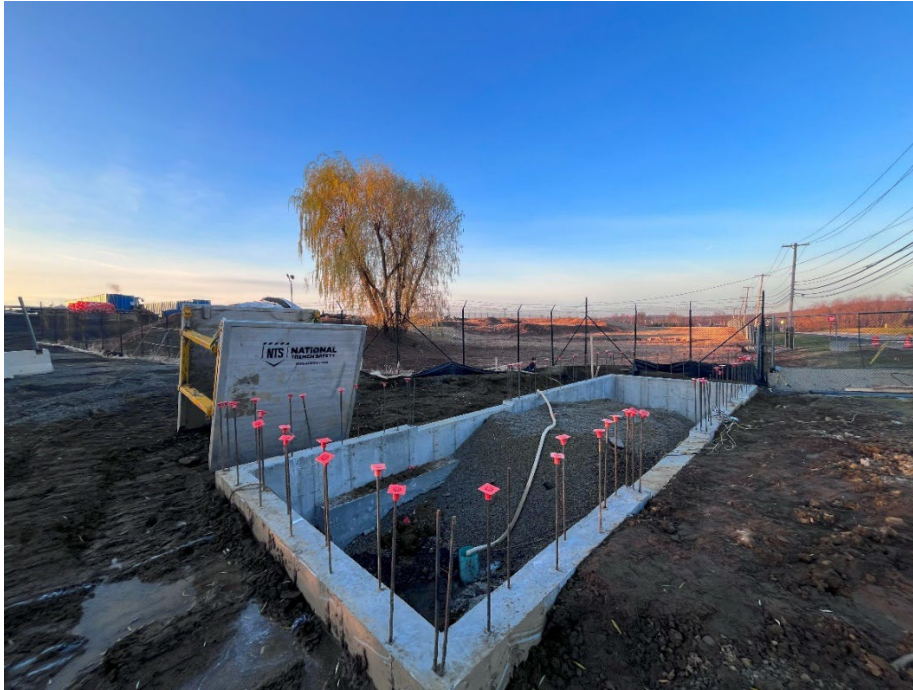
Photo 1 – Progress made as of 12/1/23. The photo shows the footing and foundation walls of the Airport Road backflow preventer building, ready for the watermain to be installed.
