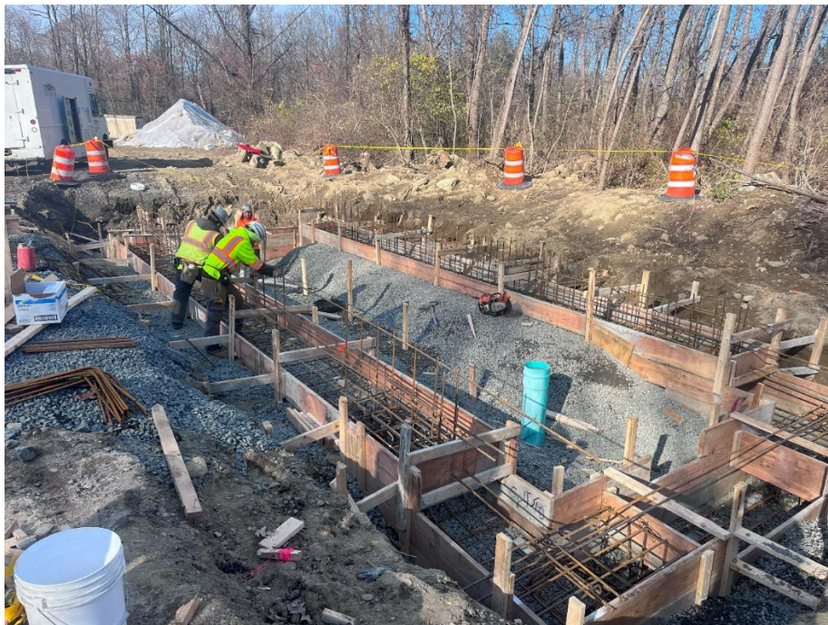
Photo 2 – Taken 11/30/23. Shows the progress made on the Tower Road backflow preventer building. Pictured is the installation of forms and rebar for the foundation footing.
