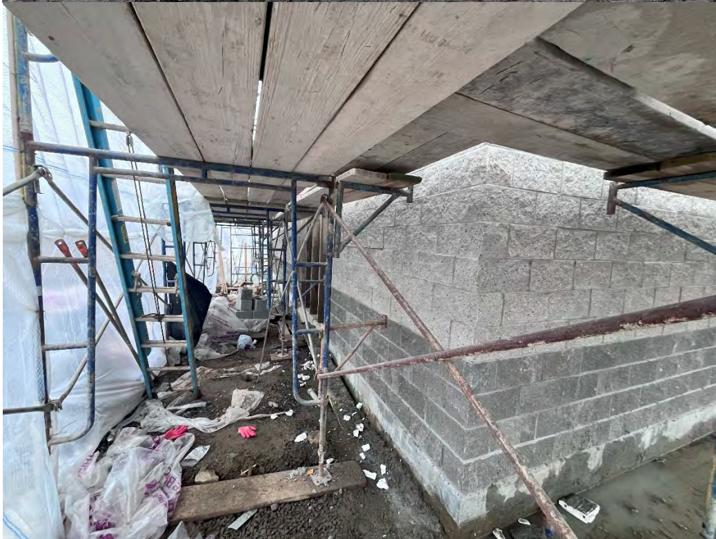
Photos 1 & 2 – Progress made as of 1/31/24. The photos show the construction progress of the stone exterior for the Airport Road backflow preventer building, as well as the surrounding scaffolding and tarp cover.
