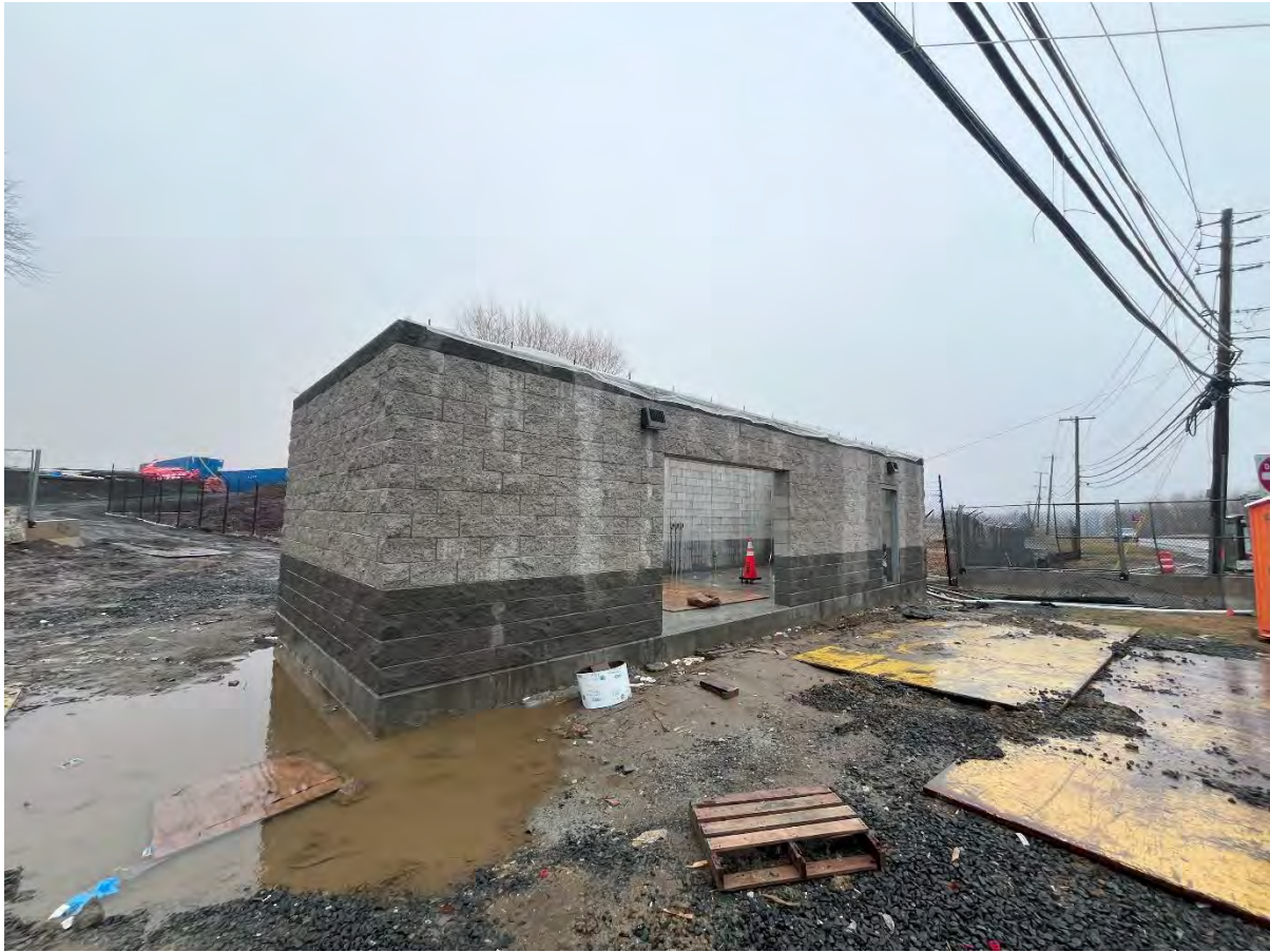
Photo 2 – Taken 2/28/24. The photo shows the construction progress of the stone exterior for the Airport Road backflow preventer building, as well as the surrounding area.
