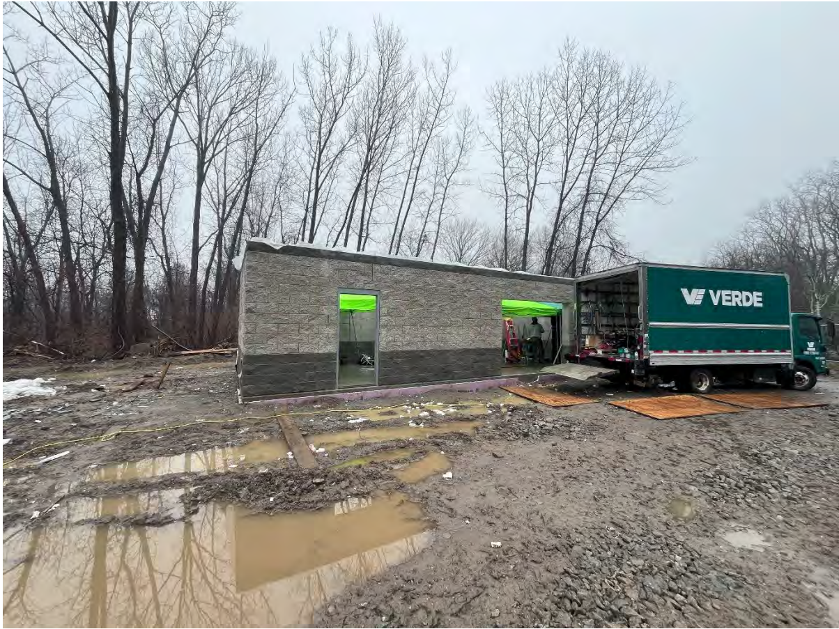
Photo 1 – Taken 2/28/24. The photo shows the construction progress of the stone exterior for the Tower Road backflow preventer building, as well as the surrounding area.
