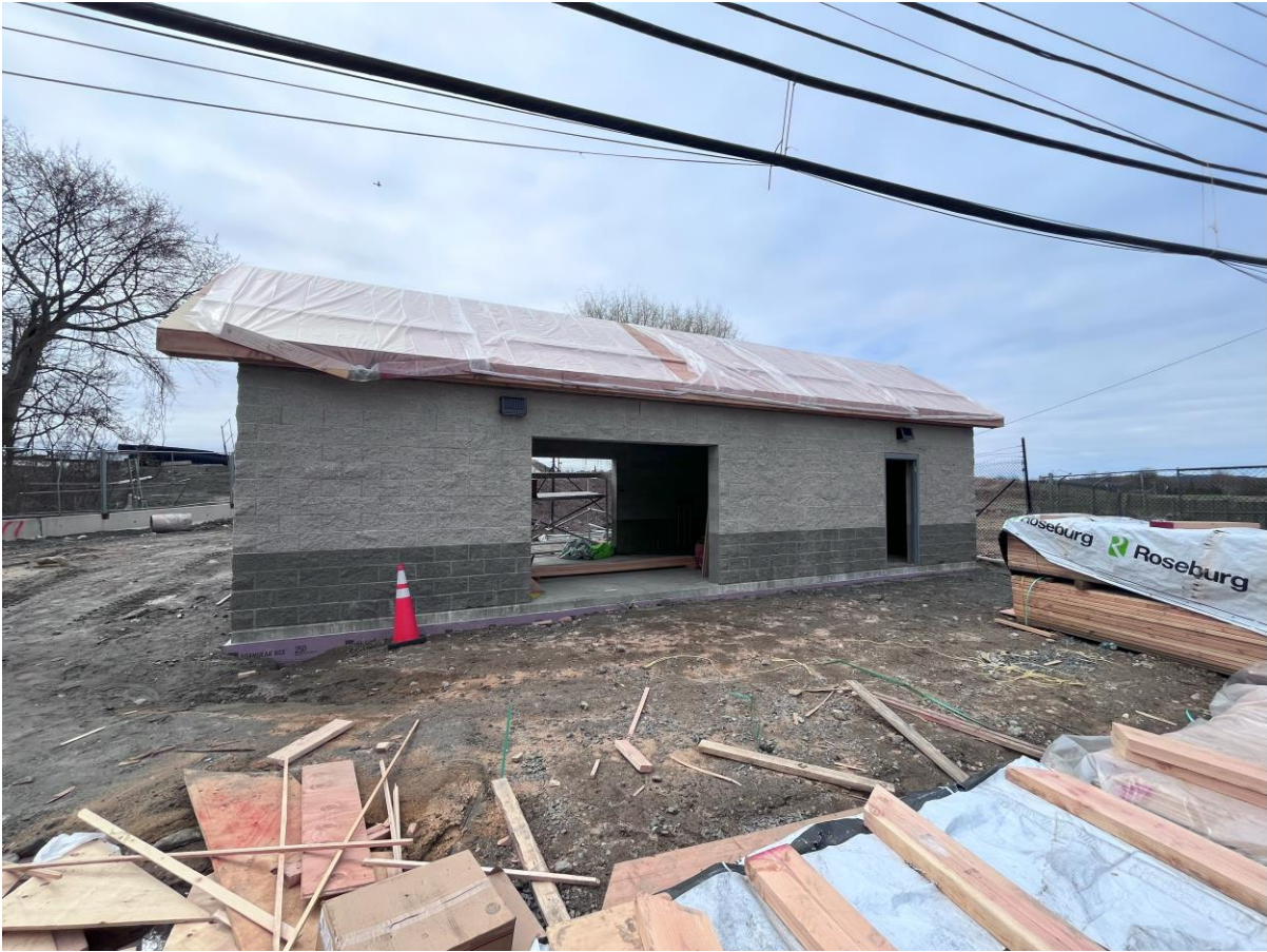
Photo 2 – Taken 3/26/24. The photo shows the construction progress of the roof for the Airport Road backflow preventer building, as well as the surrounding area.
