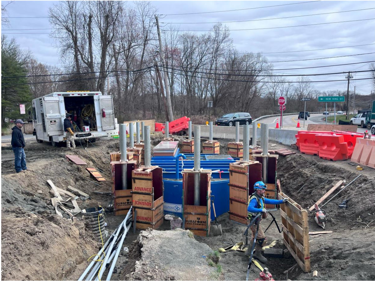
Photo 3 – Taken 3/26/24. The photo shows the RPZ meter vault after being tied into the recently installed watermain line, as well as installation of safety bollards.
