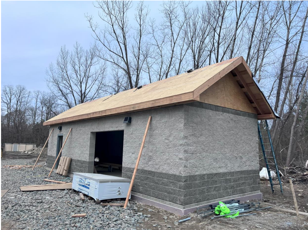
Photo 1 – Taken 3/26/24. The photo shows the construction progress of the roof for the Tower Road backflow preventer building, as well as the surrounding area.
