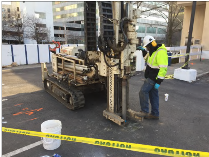
Photograph 3: Installation of 3.75-inch O.D. hollow casing at SB-14 for the installation of MW-7.
