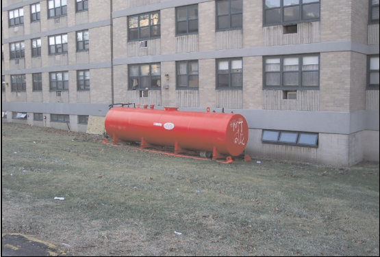
Photograph 12: 3,000-gallon AST Located at Rear of Apartment Building
