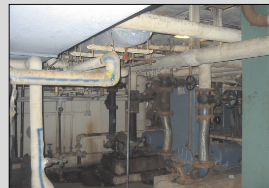
Photograph 19: Potential ACM, Pipe Insulation in Apartment Basement
