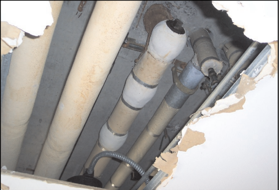
Photograph 11: Potential ACM Piping Insulation in Apartment Building
