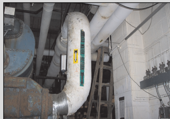
Photograph 7: Potential ACM, Piping Insulation, Mechanical Penthouse
