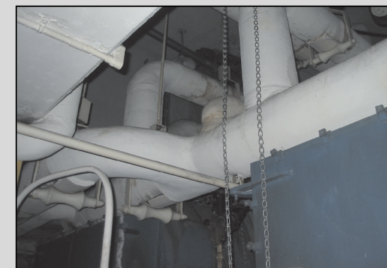
Photograph 20: Potential ACM, Pipe Insulation in Apartment Basement
