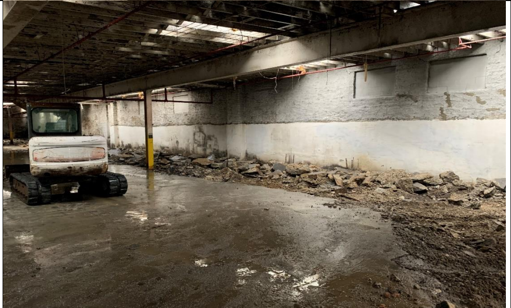
Photo 4 – View of broken up slab, facing North
