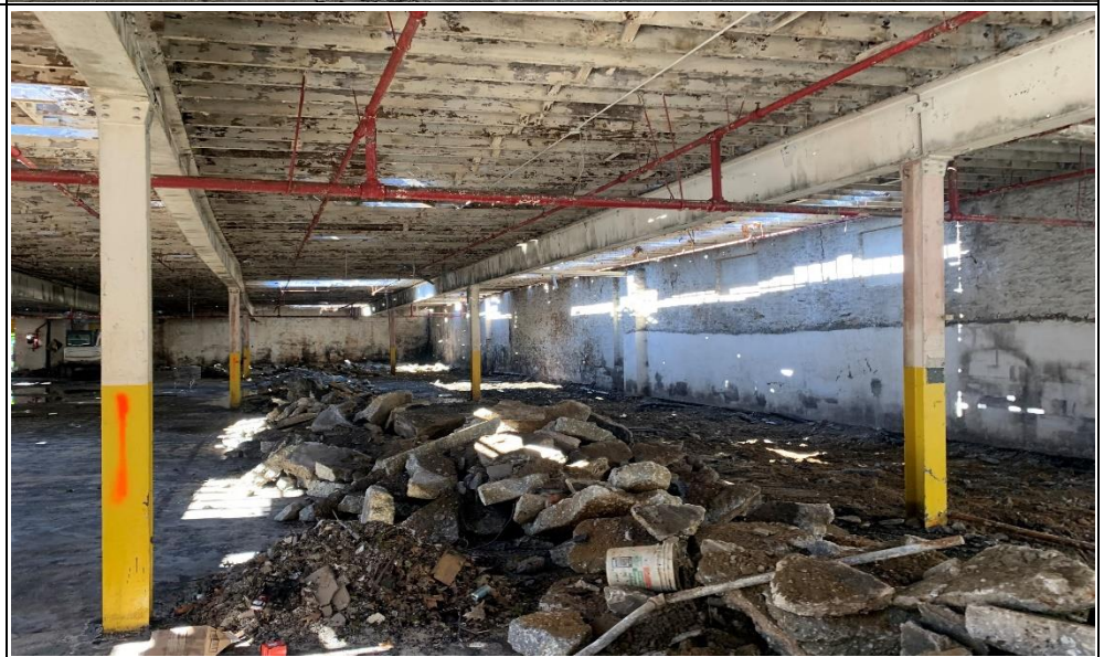
Photo 2 – View of broken slab cleared and stockpiled, facing west
