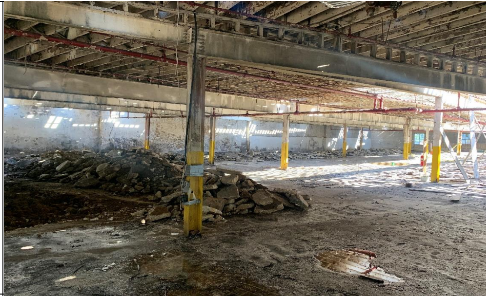
Photo 3 – View of remaining broken slab, cleared off from area. Facing North
