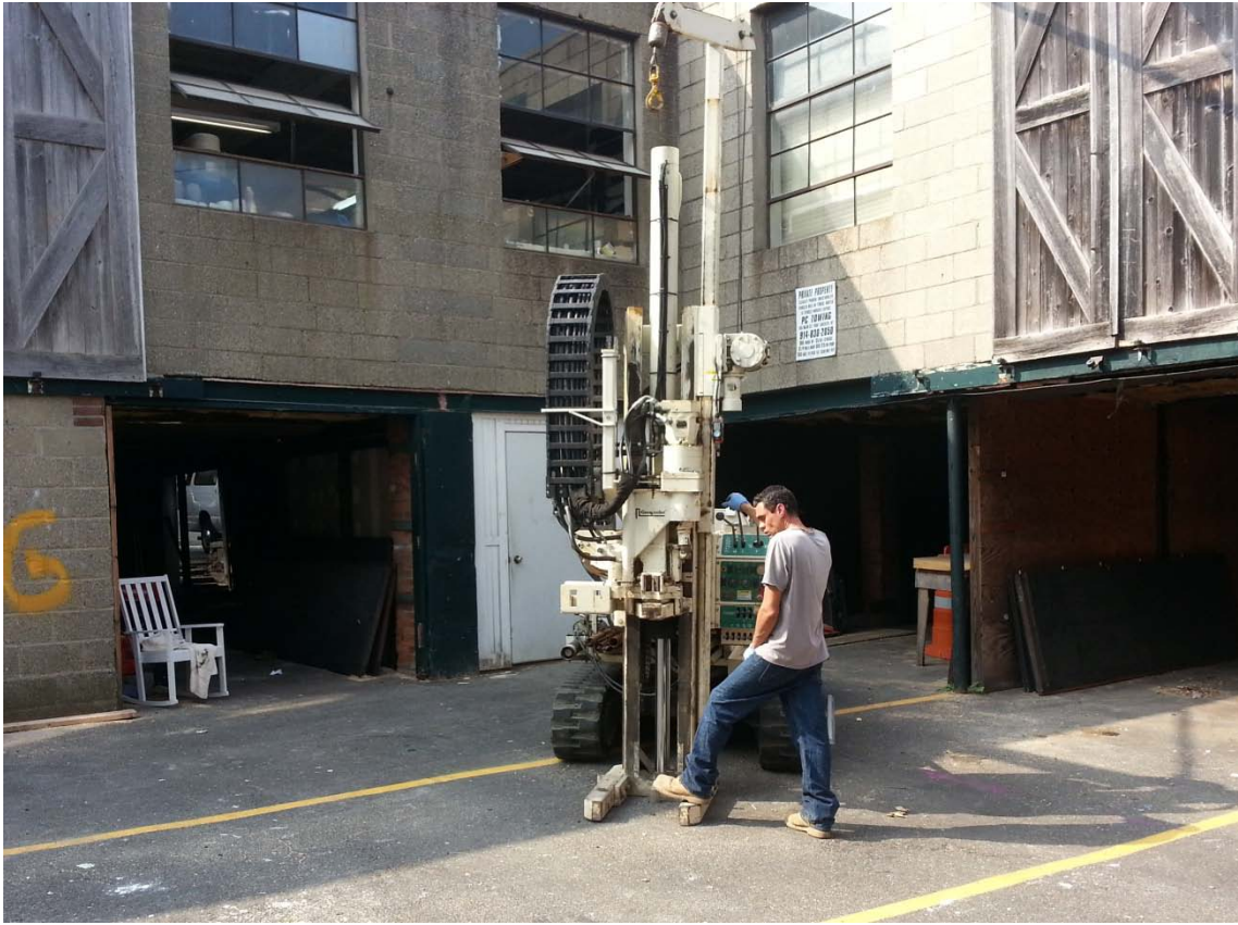
Installation of direct-push boring B-4 at the northwest portion of the Site.
