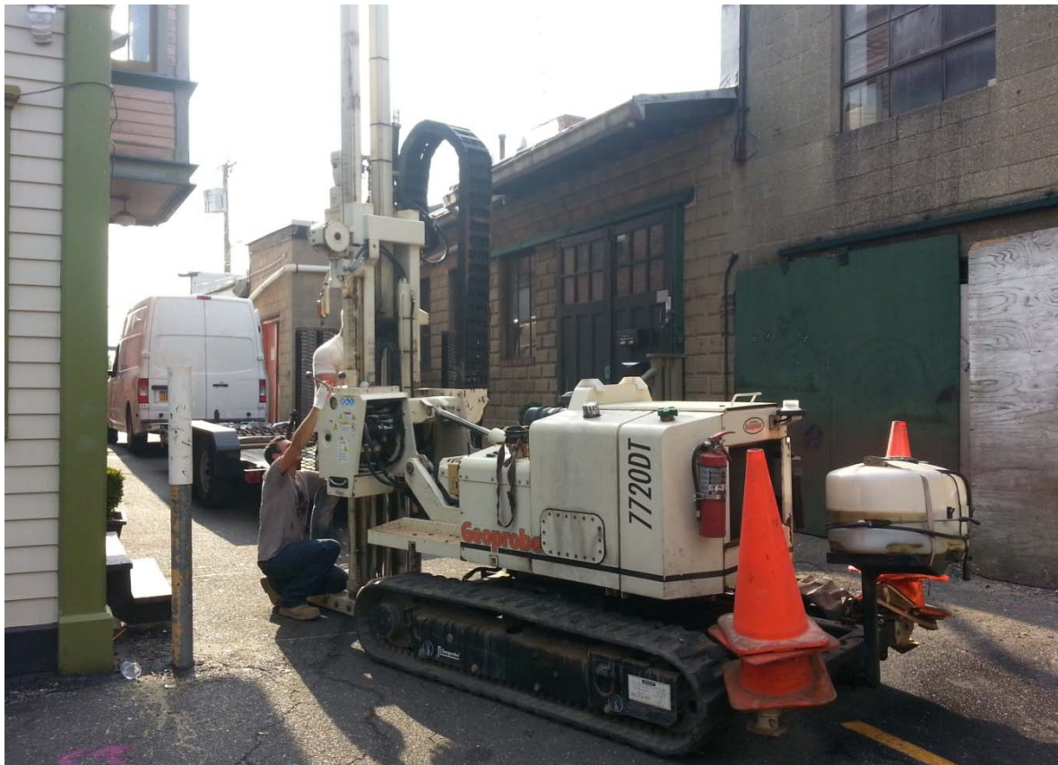
Installation of direct-push boring B-1 towards the south portion of the Site.
