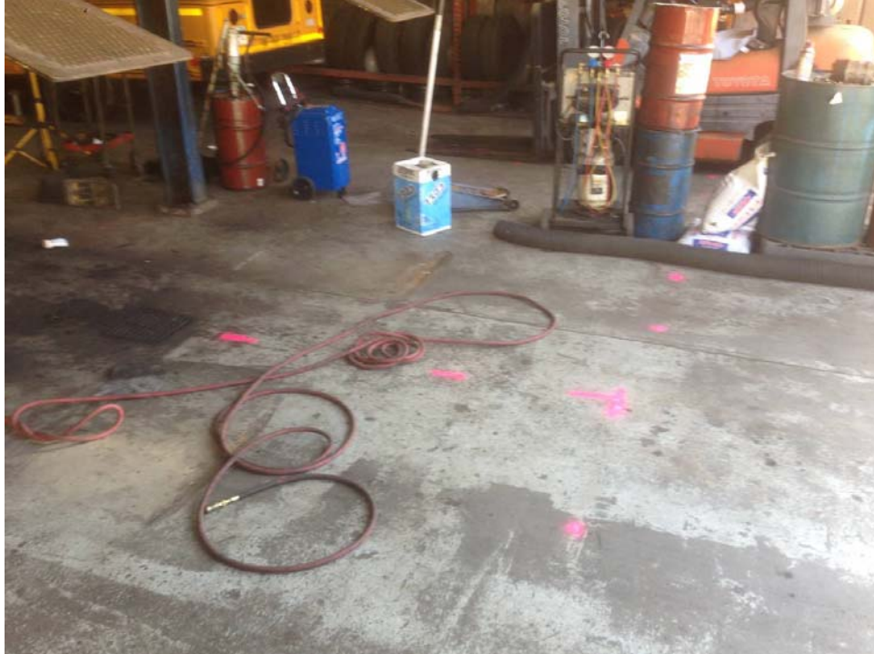
Piping from the three floor drains in the large garage was traced to the oil water separator
