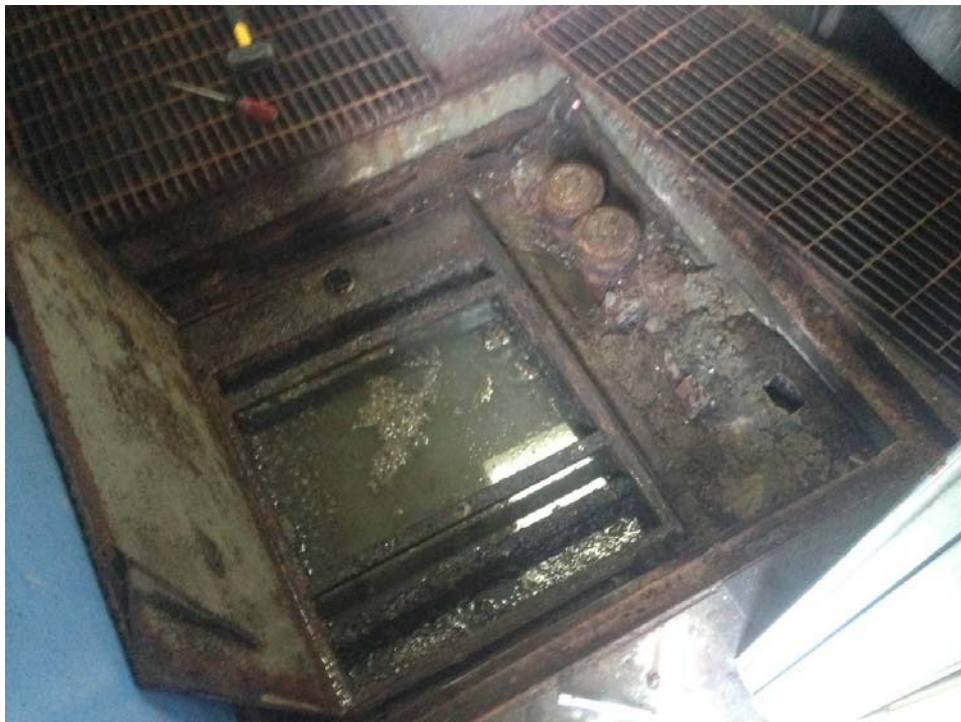
Inside the oil water separator
