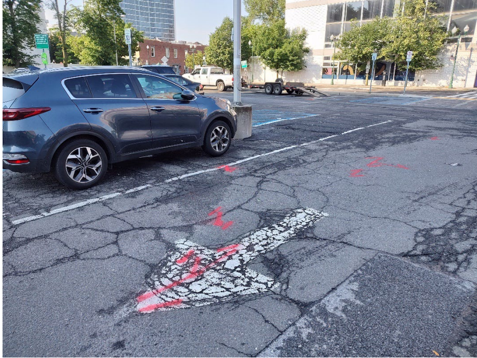
Photo 2 – View of an additional utility located within the parking lot. Electrical lines were distributed from the vault near the northeast entrance to the parking station, light poles, and continuing off the property to the southwest.
