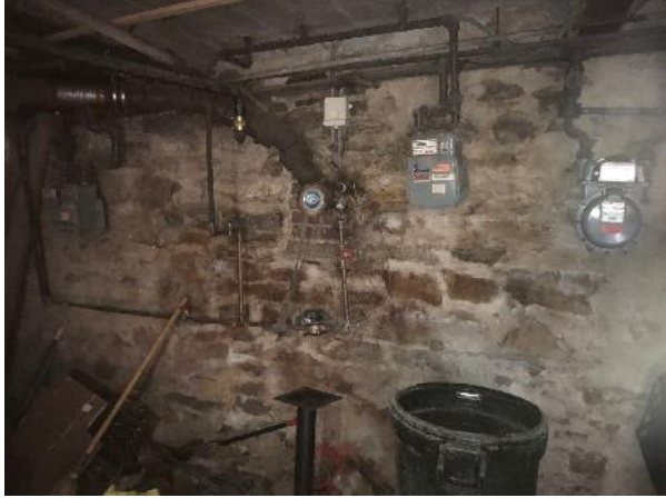
Fig. 1 : Gas / water utilities basement
