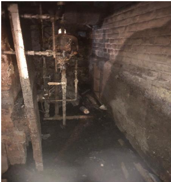
Fig. 3 : Boiler piping basement
