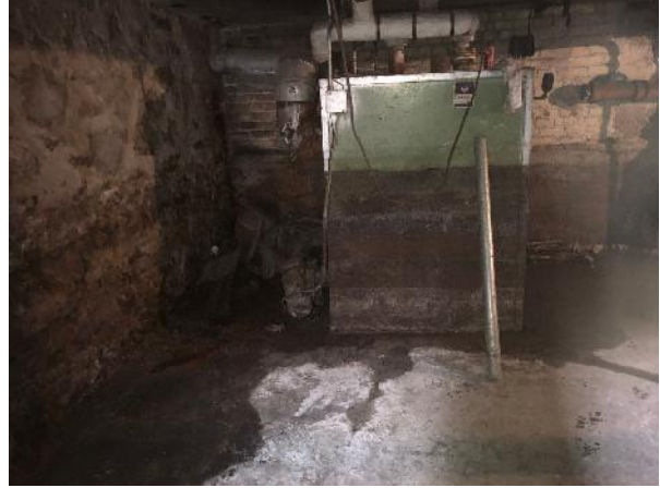
Fig. 2: Gas boiler basement
