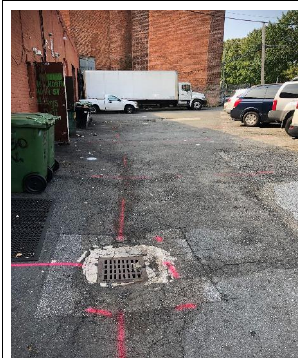
Fig. 5. Drainage rear parking lot
