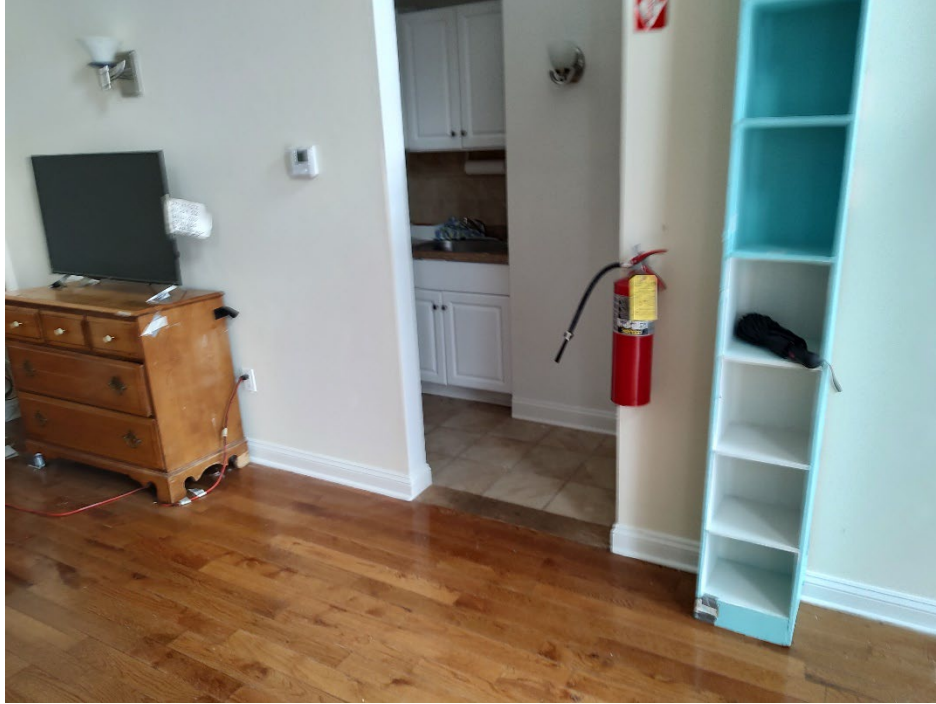
Photo 2 – View of the residential building behind the office which contained a floating floor (floor resting on rafters instead of on the soil surface).
