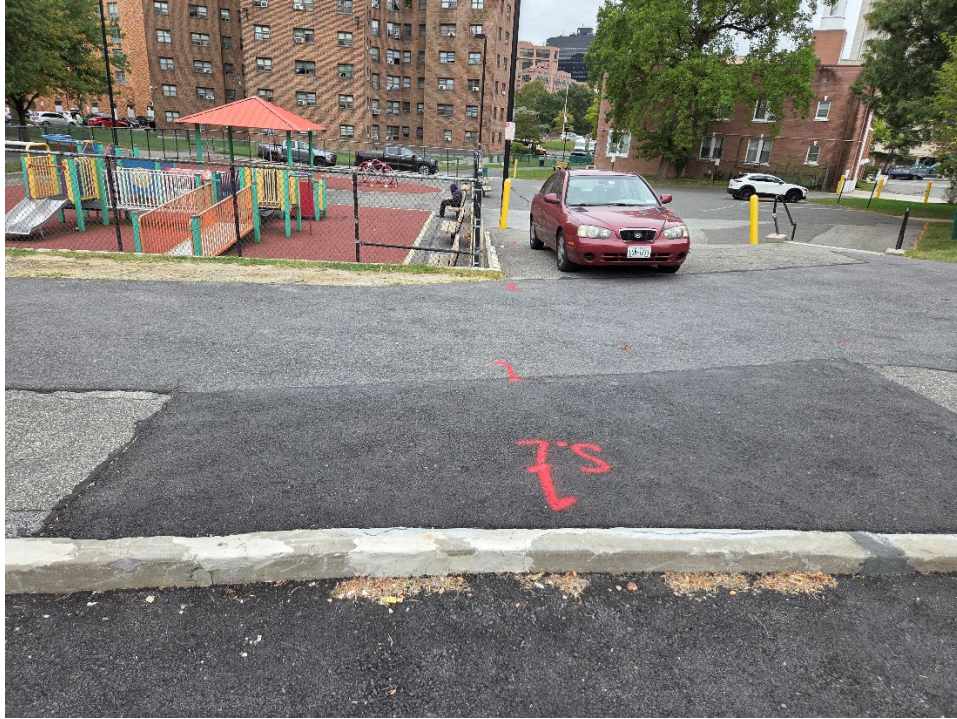
Photo 1 – View of a portion of the site with an electrical site lighting line marked in red.
