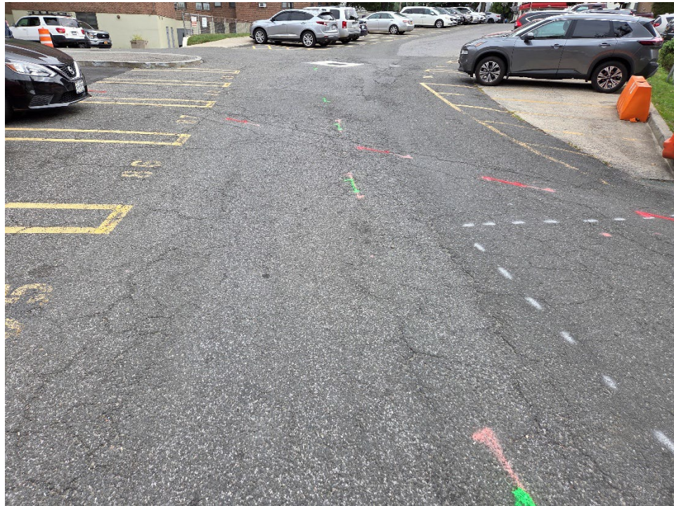
Photo 4 – Multiple drainage lines were detected in the parking lot, all marked in green leading to the storm drains.
