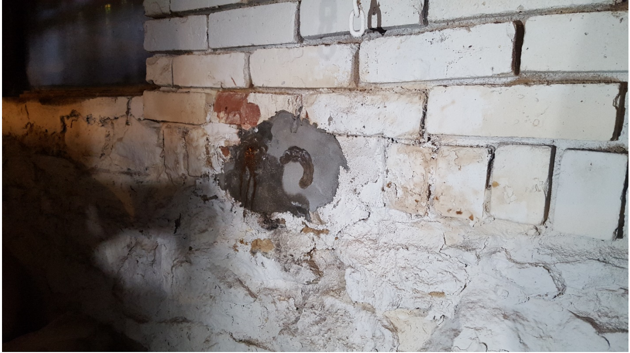
Photo 1 Patched holes in basement opposite exterior northern fill and vent pipes.
