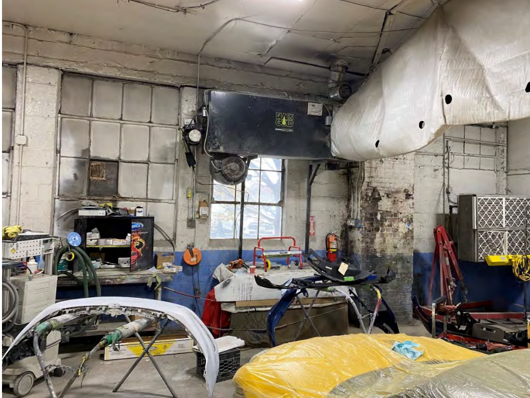
P.29 Auto Repair Shop – Waste Oil Burner
