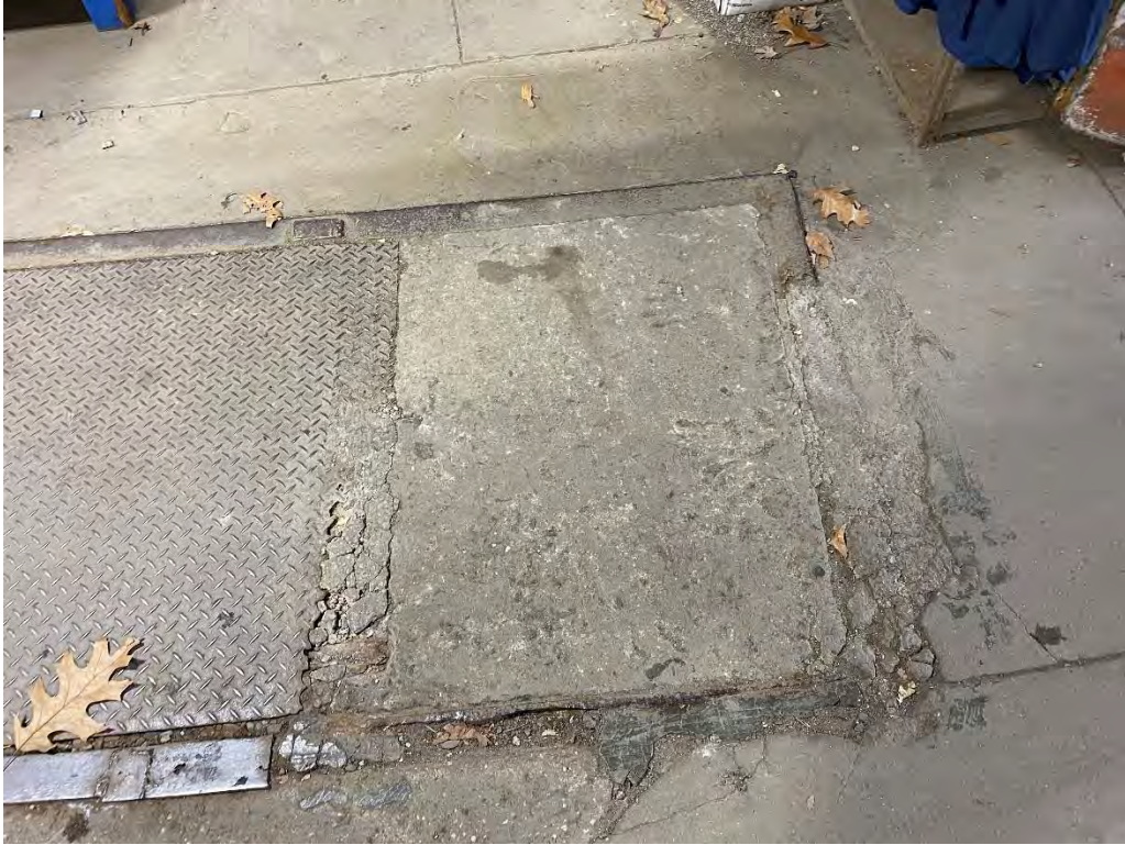
P.39 Auto Repair Shop – Floor Anomaly (Possible Previous Pit)
