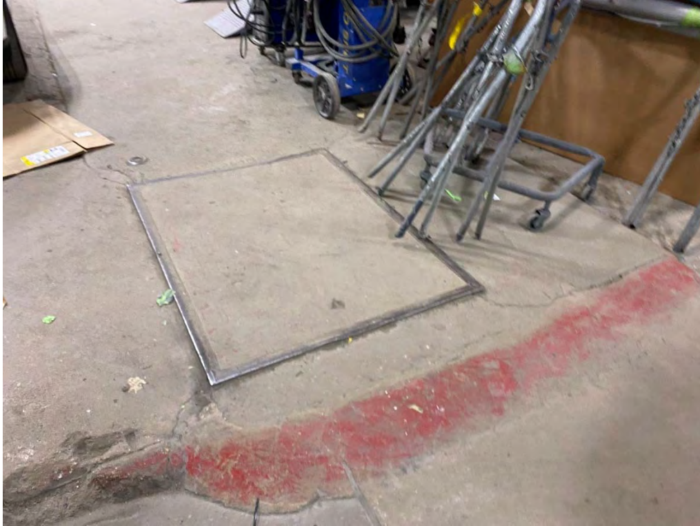
P.37 Auto Repair Shop – Floor Anomaly
