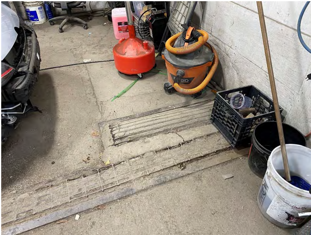
P.32 Auto Repair Shop – Filled Floor Drains
