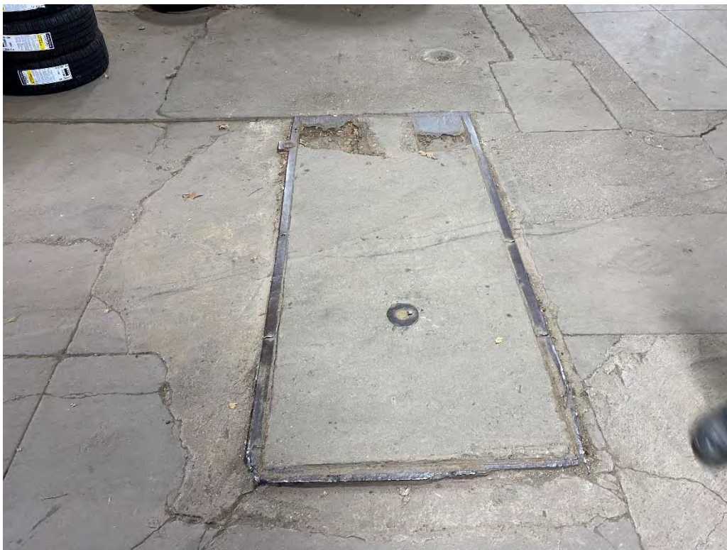
P.36 Auto Repair Shop – Floor Anomaly
