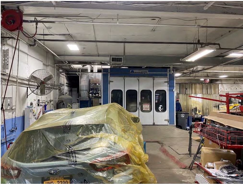
P.40 Auto Repair Shop – Paint Booth
