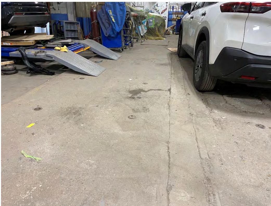
P.33 Auto Repair Shop – Filled Floor Drains
