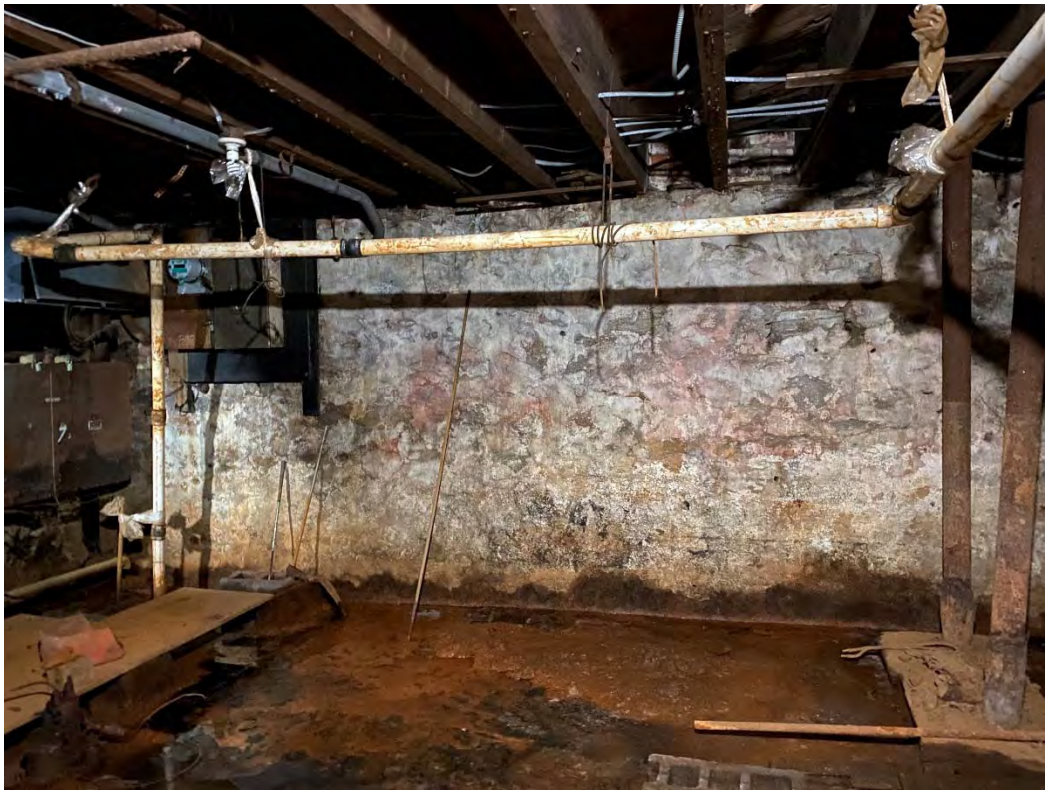
P.16 Magic Touch Cleaners – Sump Pump Piping
