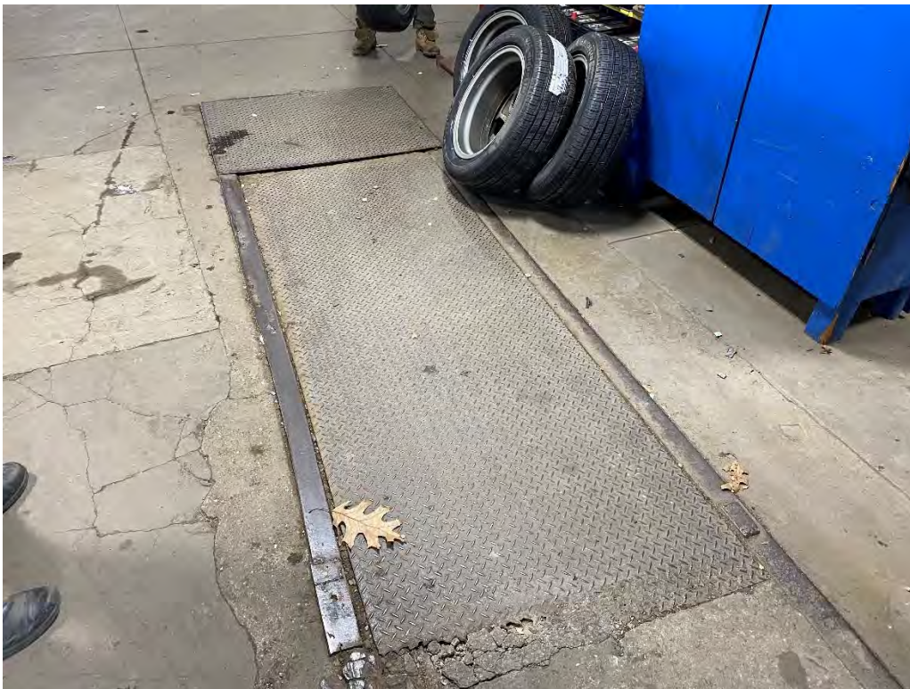
P. 38 Auto Repair Shop – Floor Anomaly (Possible Previous Pit)
