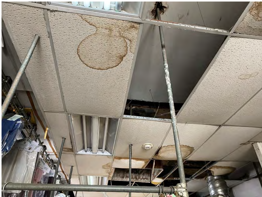
P.6 Magic Touch Cleaners - Damaged Ceiling Tiles
