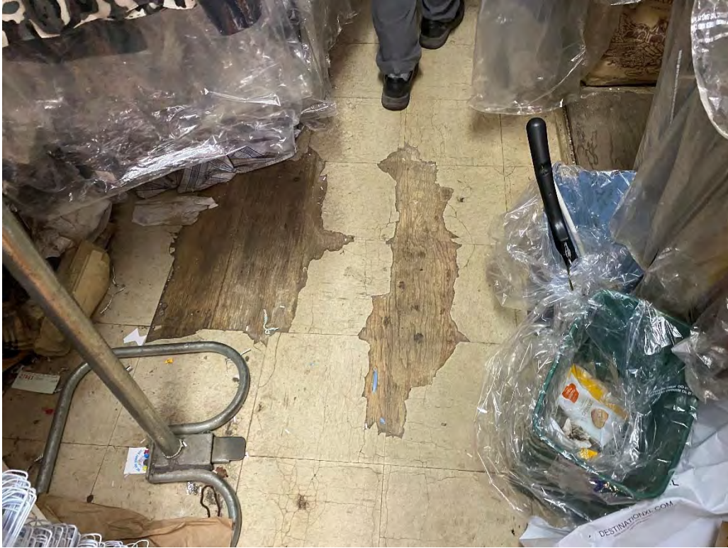
P. 5 Magic Touch Cleaners - Damaged Floor Tiles
