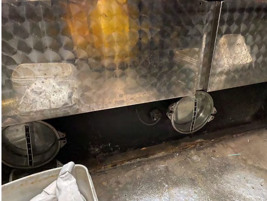
P.9 Magic Touch Cleaners - Main Dry Cleaner Cleaning Fluid Containment
