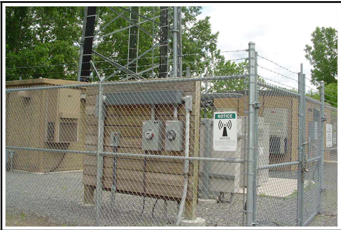
Photo #4 Description: View of Crown Castle wireless telecommunications area located on the northeastern portion of the site.
