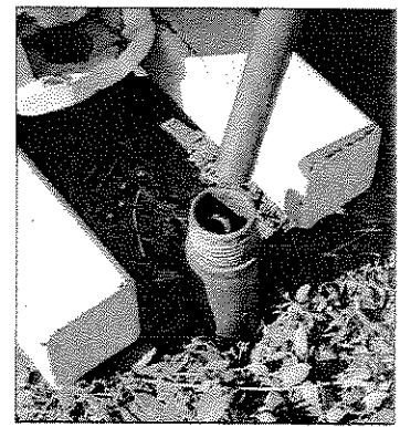
Figure 4.23. Thread a 1.0-inch probe rod onto inner rod string to retrieve filled liner.
