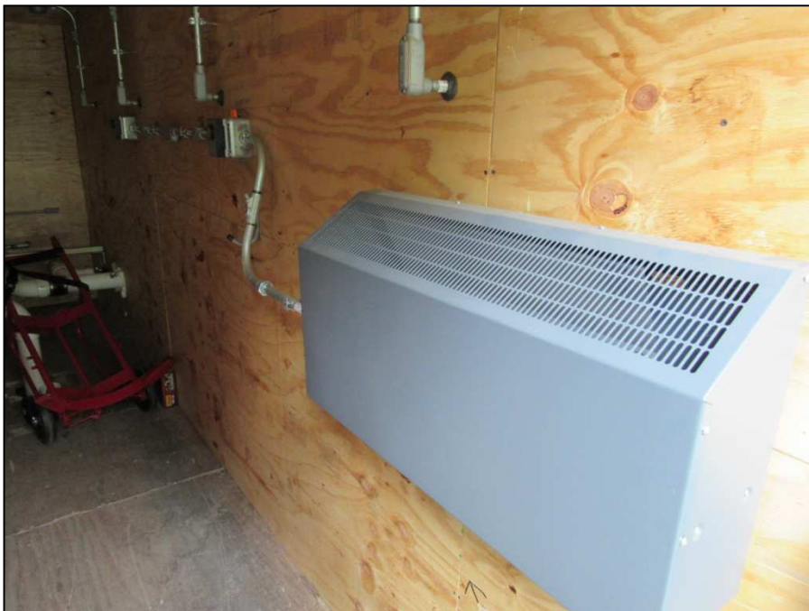
Electric heater for heating the SVE shed, connected to a thermostat.
