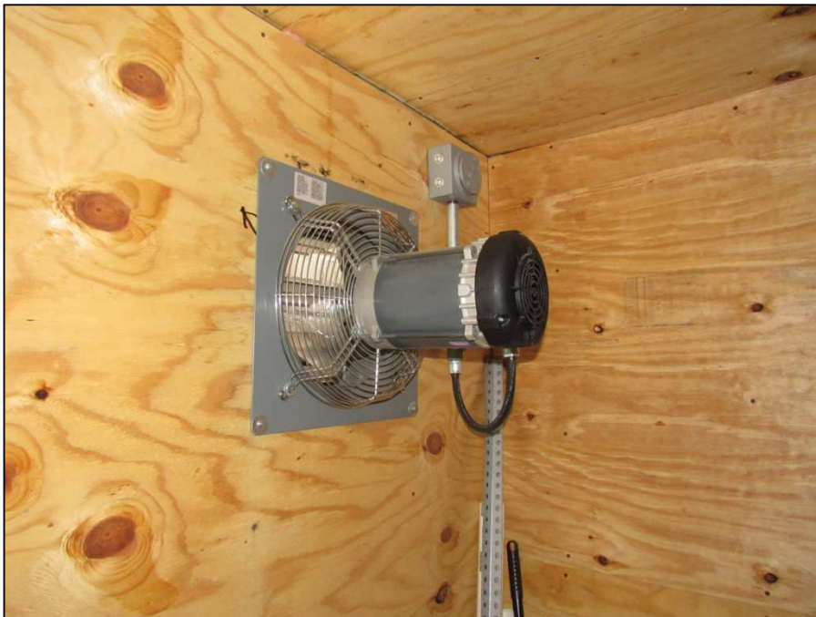
SVE Shed exhaust fan connected to a thermostat for cooling the shed.
