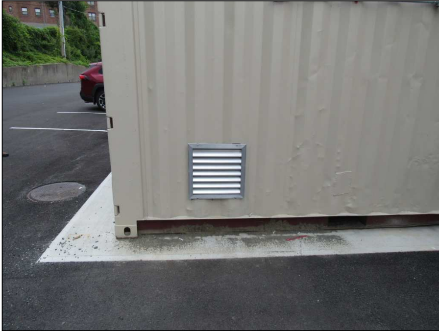
Air intake grate for bringing cooler air into shed when exhaust fan operates.
