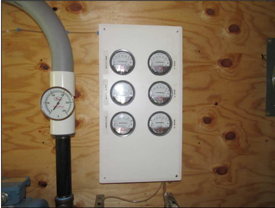
System effluent air temperature gauge and pressure gauges for each SVE well, pre and post air filter, and post blower effluent line.
