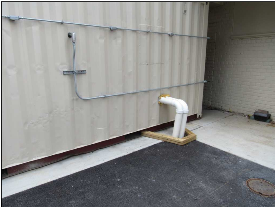
Extraction wells SVE-1 and SVE-2 conveyance piping rising above ground and entering the SVE shed.
