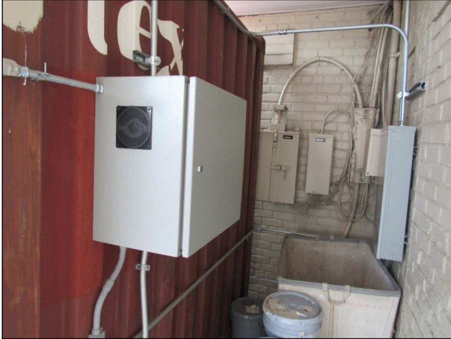
Electrical supply box housing the shed electrical supply and the variable frequency drive (VFD) for the SVE blower.
