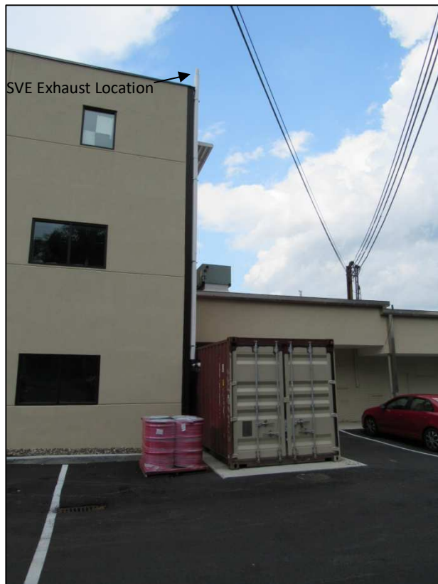
SVE shed with exhaust pipe exiting and exhausting above the adjacent high roof.
