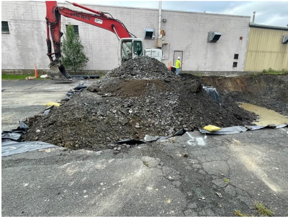
Photograph 17: Hazardous soil stockpiled within lined portion of IRM excavation area pending loading for offsite disposal. View looking south. (Photo taken 9/10/21).
