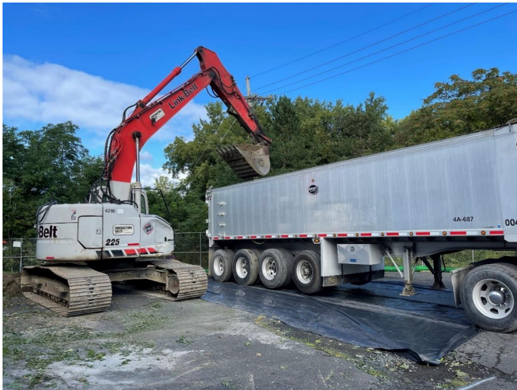
Photograph 9: Excavation and loading of non-hazardous soil for offsite disposal at the Green Ridge Landfill in Gansevoort, NY. View looking northwest. (Photo taken 9/3/21).
