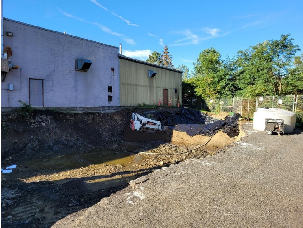
Photograph 25: Dewatered excavation area prior to placement of additional approved backfill. Remediation contact water was pumped to temporary holding tanks pending characterization and offsite disposal. View facing southwest. ( Photo taken 9/21/21).
