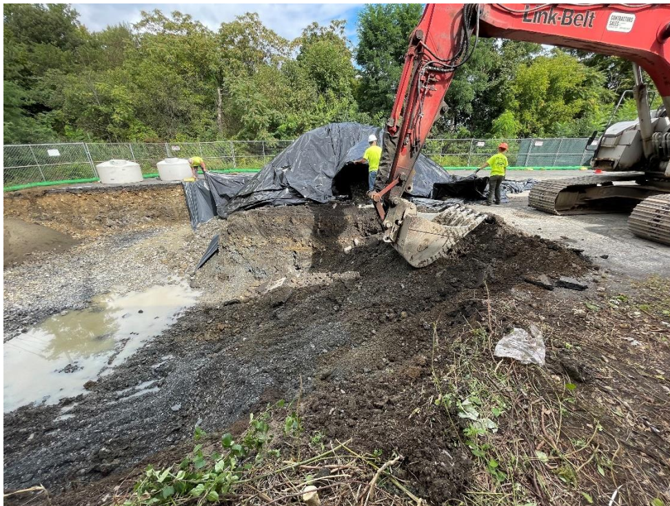
Photograph 18: Placement of poly sheeting over temporarily stockpiled hazardous soil within lined portion of IRM excavation area pending loading for offsite disposal. View looking north. (Photo taken 9/10/21)
