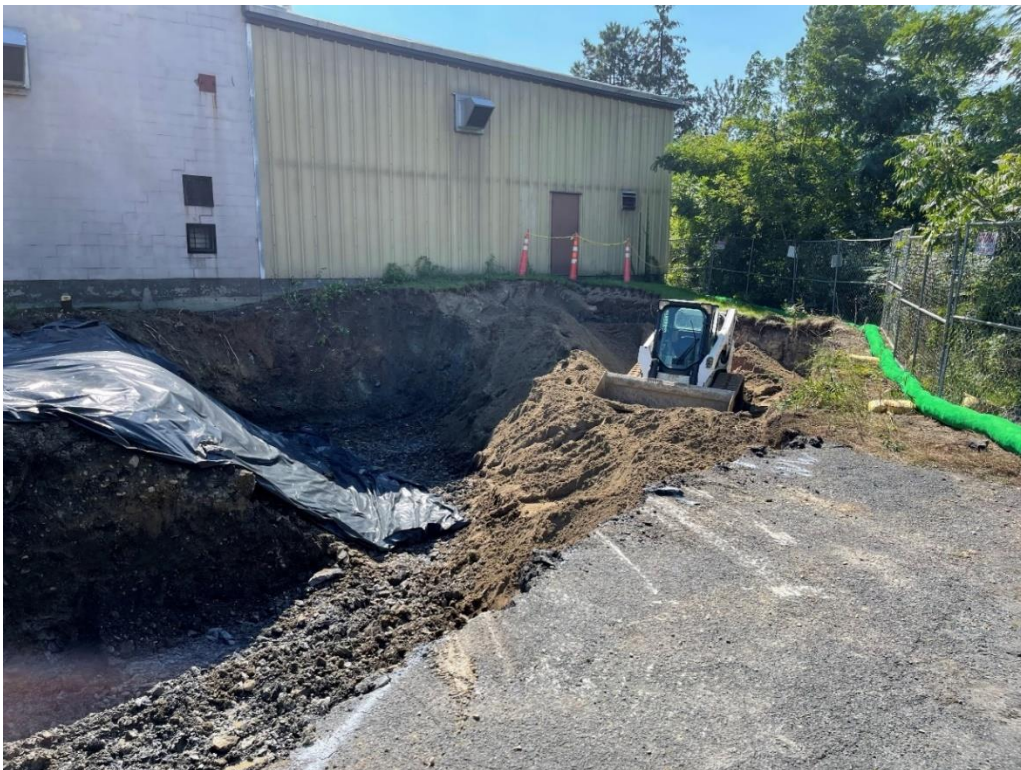
Photograph 12: Placement of approved backfill in completed excavation area. Poly sheeting placed over impacted soil to prevent cross contamination. View facing southwest. (Photo taken 9/8/21).
