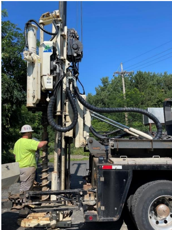
Photograph 3: Abandonment of Monitoring Wells MW-2S and 5S within the IRM soil excavation area. View looking west-northwest. (Photo taken 7/23/21).
