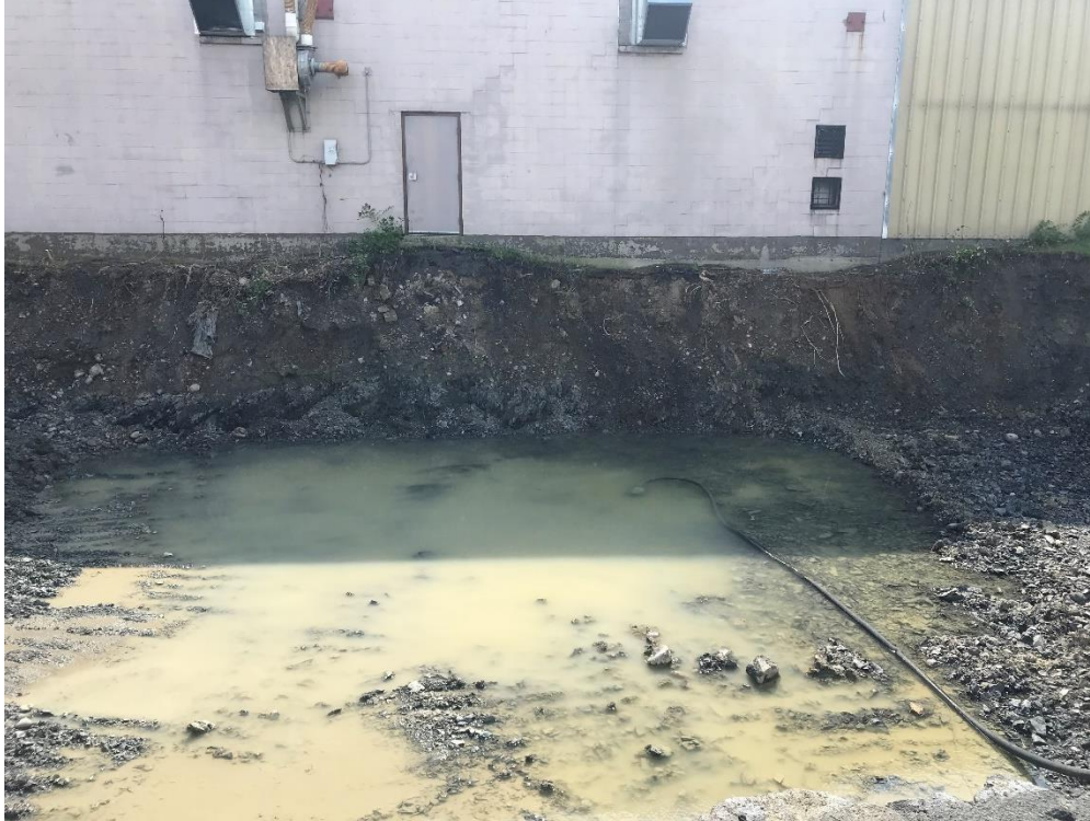
Photograph 23: Excavation floor completed to two feet into weathered bedrock surface within central portion of IRM excavation area. Accumulated remediation contact water prepared to be pumped to temporary holding tanks pending characterization and offsite disposal. View facing south. ( Photo taken 9/15/21).
