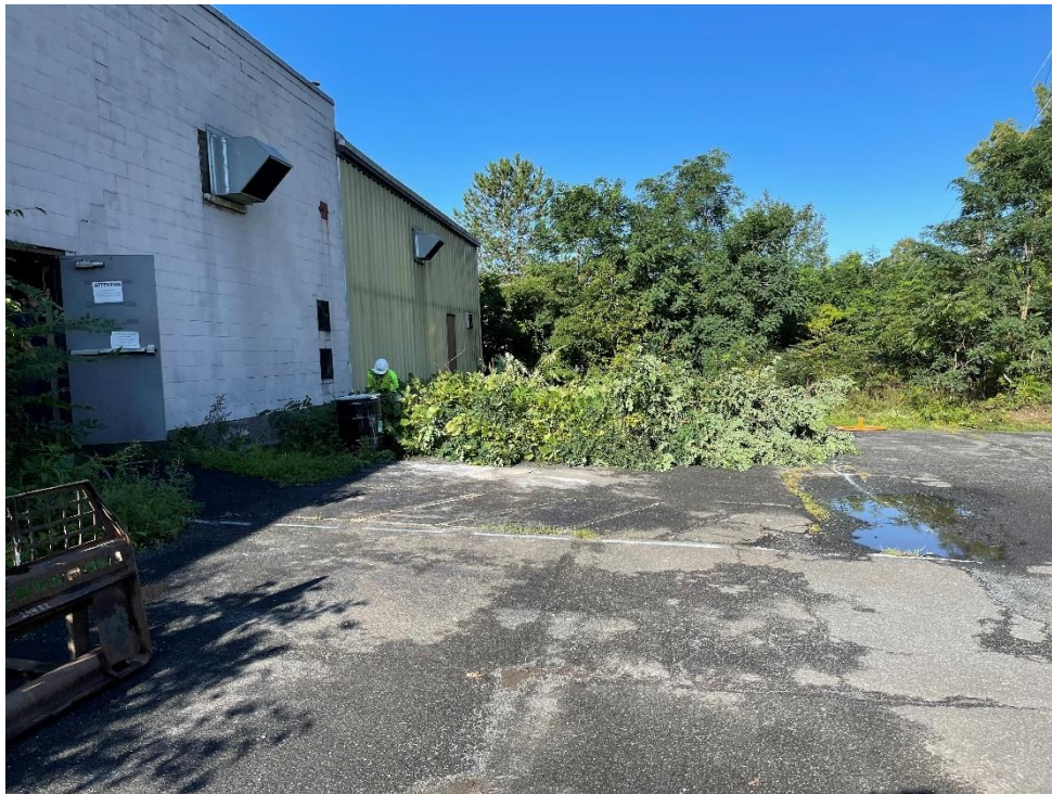
Photograph 6: Site Preparation – vegetation removal within soil excavation limits. View looking west. (Photo taken 9/2/21).
