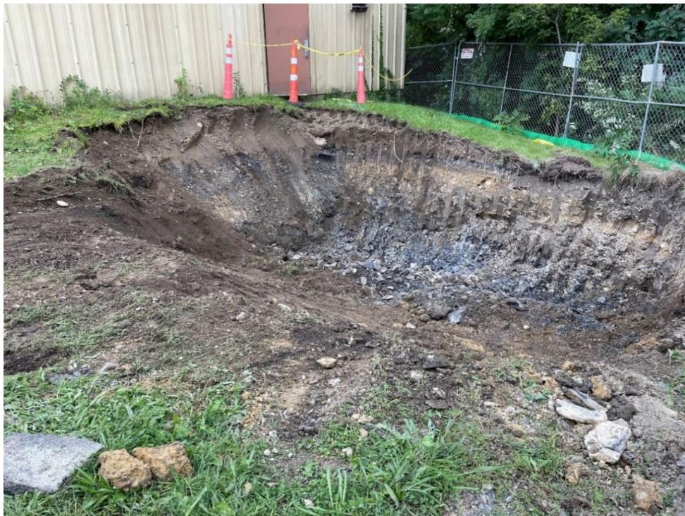
Photograph 10: Excavation of non-hazardous soil in southwest portion of the IRM excavation area. Excavation sidewall was sloped along the building to protect its foundation. View looking southwest. (Photo taken 9/3/21).
