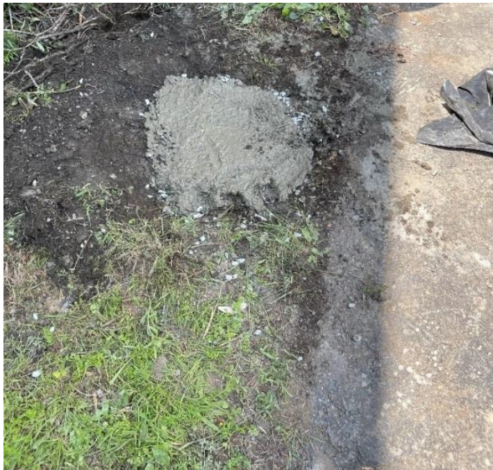
Photograph 4: Representative view of completed abandonment of Monitoring Well MW-5S. View looking west. (Photo taken 7/23/21).
