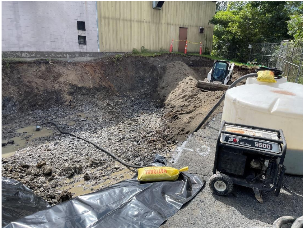
Photograph 19: Removal of remediation contact water with visible sheen from the hazardous soil excavation area for temporary storage pending characterization and offsite disposal. View looking southwest. (Photo taken 9/10/21)
