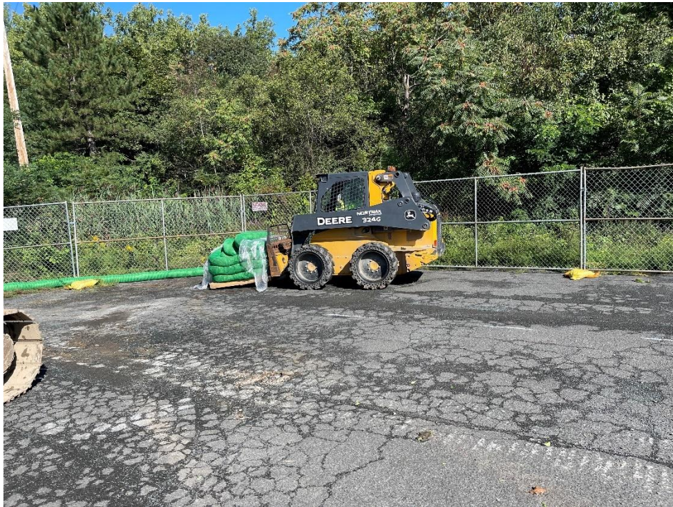
Photograph 7: Site Preparation – Installation of perimeter fencing and erosion controls. View looking northwest. (Photo taken 9/2/21).
