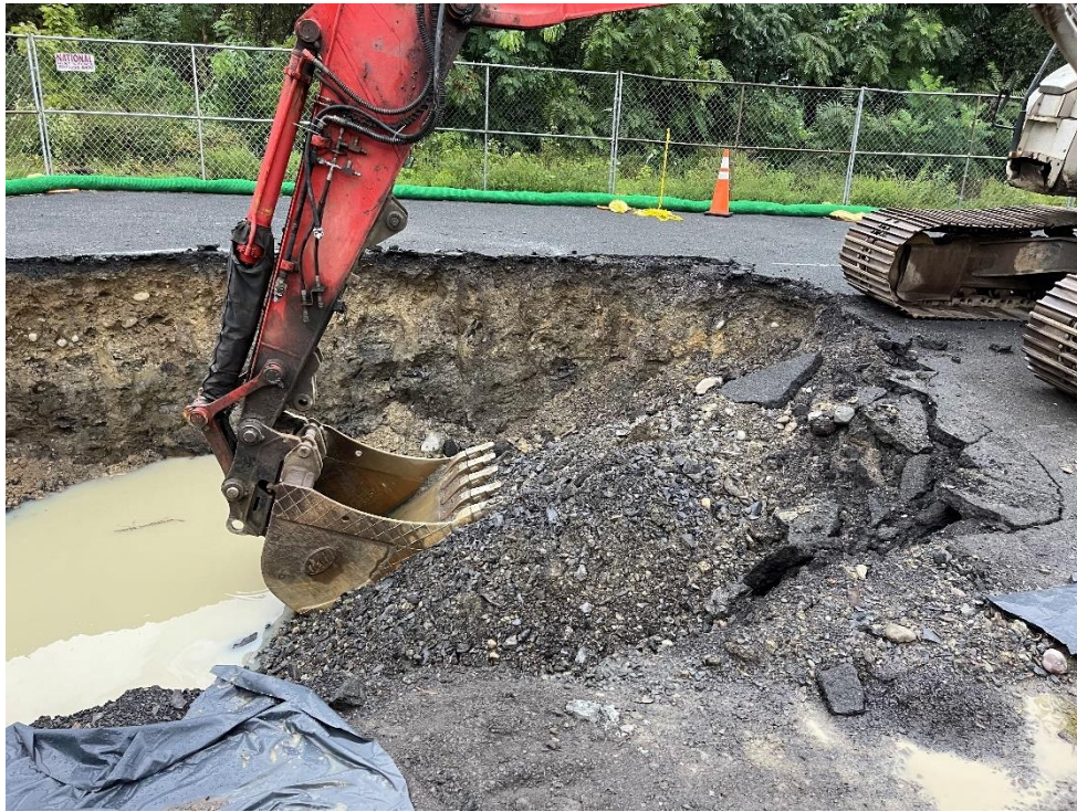
Photograph 13: Excavation of non-hazardous soil along the northern limit of the IRM excavation area. View looking north. (Photo taken 9/8/21).
