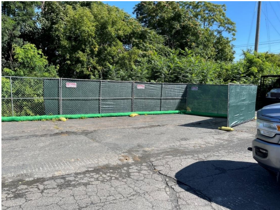
Photograph 8: Site Preparation – Installed perimeter fence and erosion controls. View looking northeast. (Photo taken 9/2/21).
