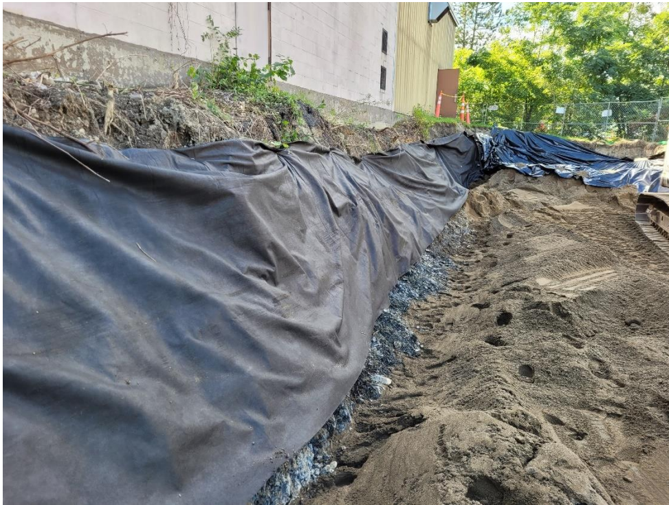
Photograph 29: Geotextile fabric demarcation layer between unexcavated soil beneath building foundation and clean backfill. View facing west. (Photo taken 9/21/21).
