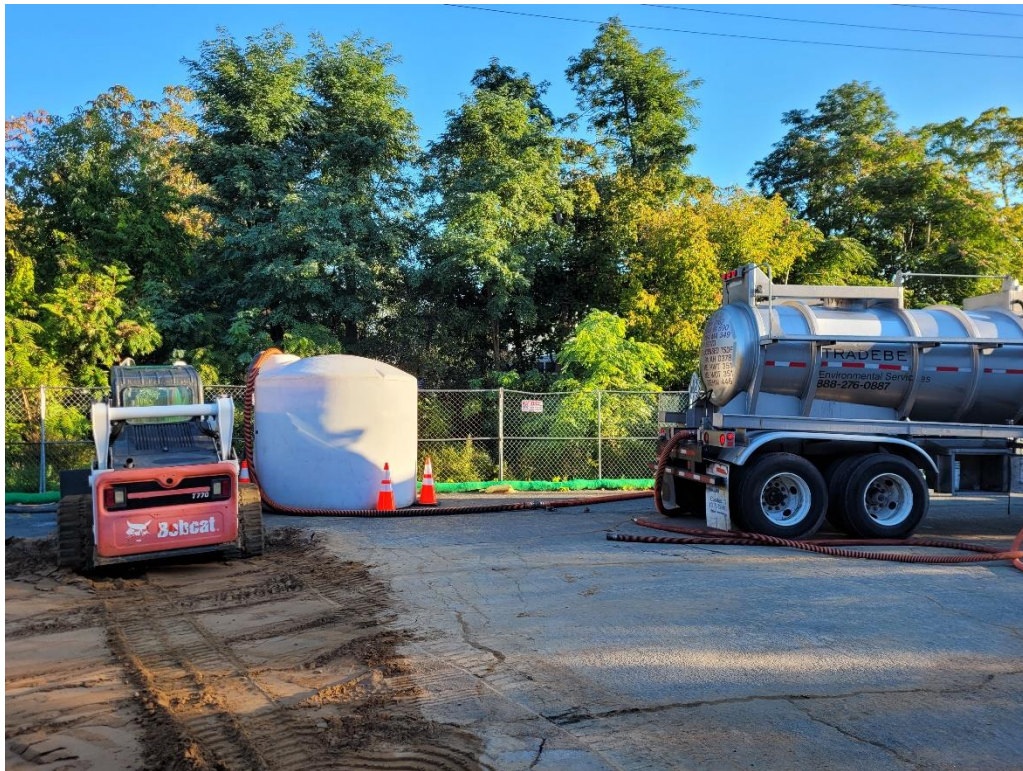
Photograph 32: Removal of remediation contact water from onsite holding tanks for disposal by Tradebe Treatment and Recycling, LLC. View facing north. (Photo taken 10/1/21).
