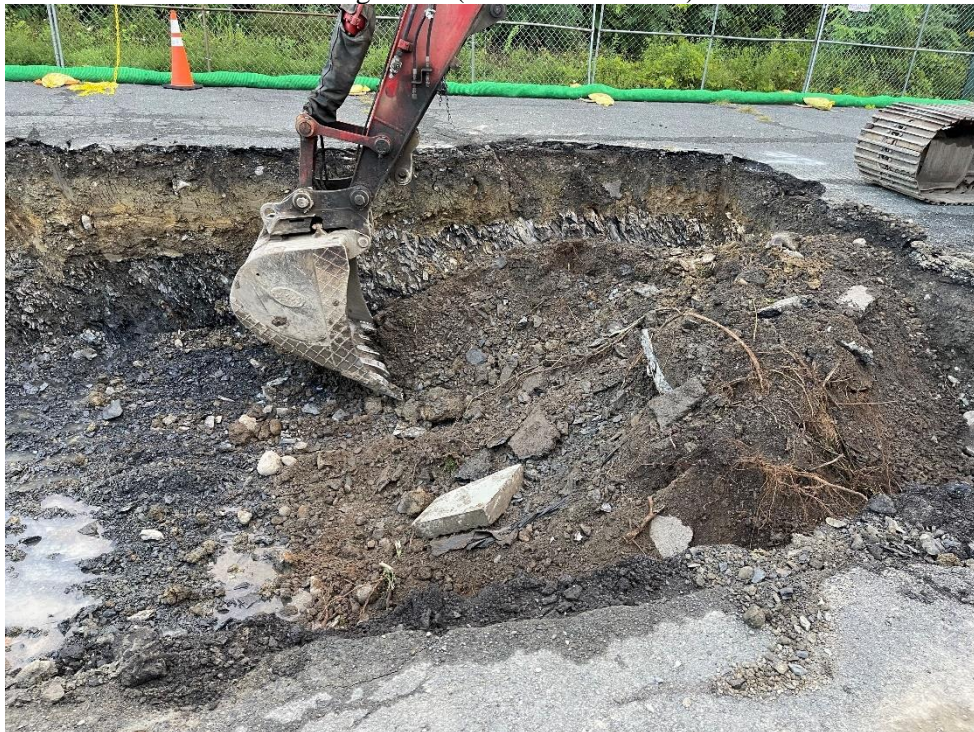
Photograph 14: Excavation of non-hazardous soil up to the northeastern limit of the IRM excavation area. View looking northeast. (Photo taken 9/10/21).
