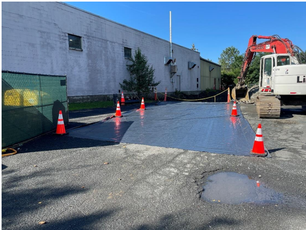
Photograph 20: Representative photograph of prepared truck loading area to prevent tracking of excavated soil. View facing west-southwest. (Photo taken 9/13/21).
