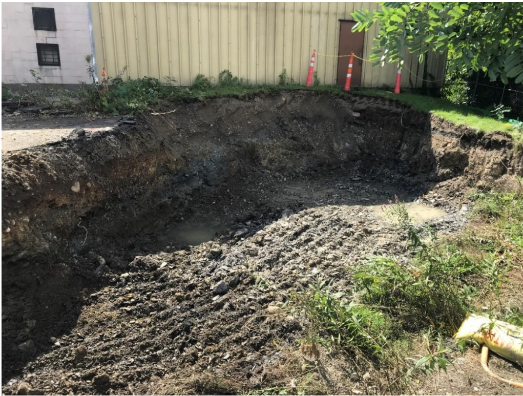
Photograph 11: Completed excavation of non-hazardous soil and weathered bedrock in the southwest portion of the IRM excavation area. View looking southwest. (Photo taken 9/7/21).
