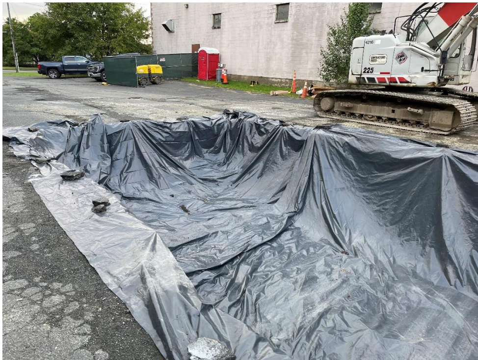
Photograph 16: Lined area within IRM excavation area limits to stockpile hazardous soil to facilitate truck loading. View looking east-southeast. (Photo taken 9/10/21).
