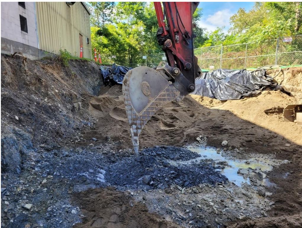
Photograph 28: Location of attempted excavation of competent bedrock for visual assessment and sample collection. Excavation was unsuccessful and rock sample collected with a drill rig on 10/8/21. View facing west. (Photo taken 9/21/21).
