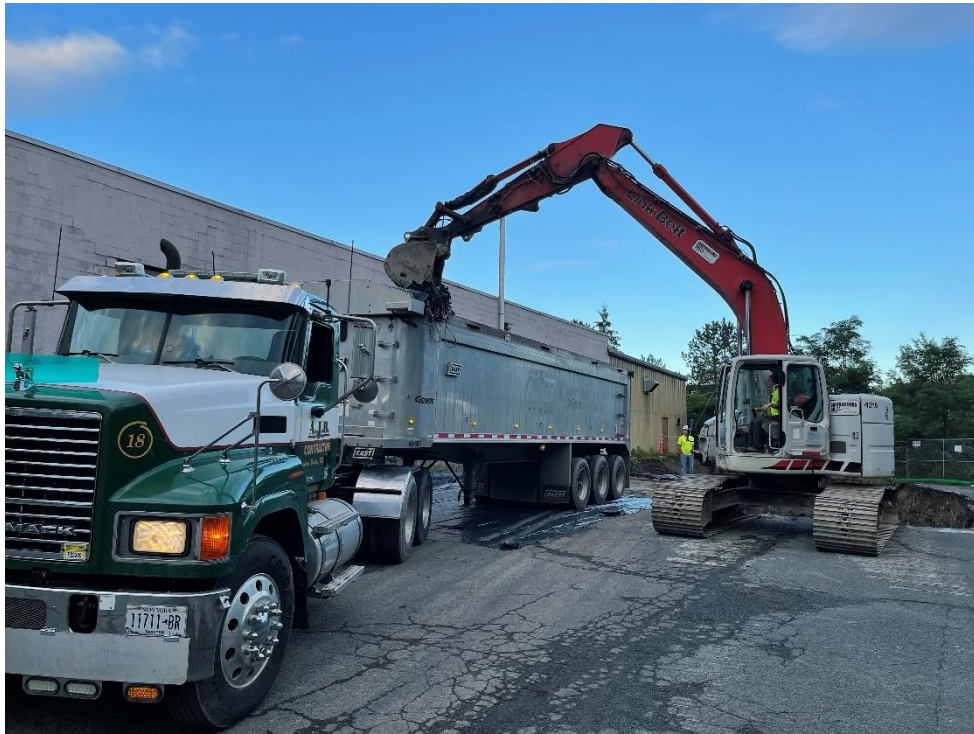
Photograph 15: Representative photograph of loading non-hazardous soil for offsite disposal. View looking west-southwest. (Photo taken 9/10/21).
