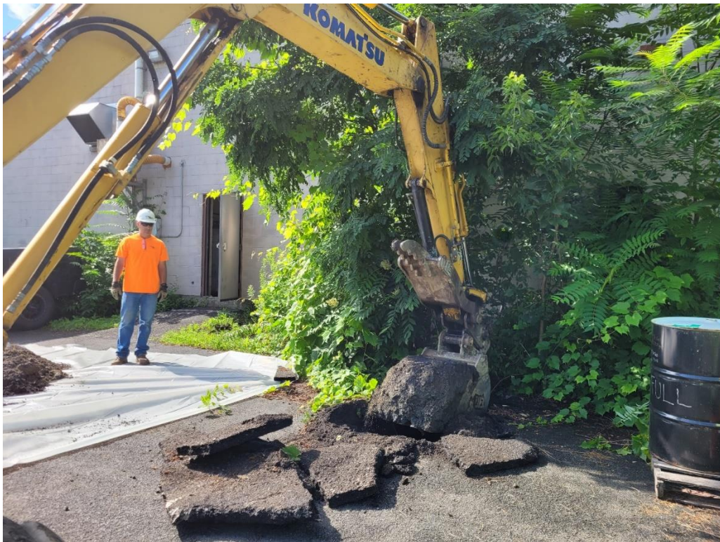
Photograph 2: Test Pit for collection of hazardous waste characterization sample. View looking southeast. (Photo taken 7/4/21).
