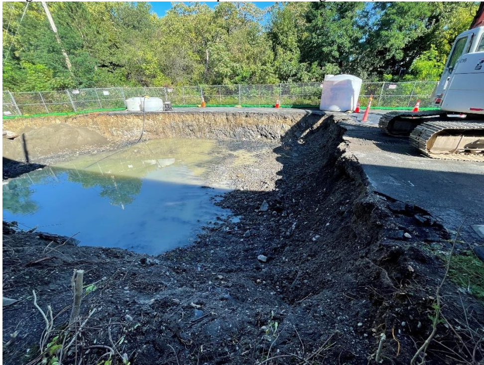
Photograph 24: Excavation floor completed to two feet into weathered bedrock surface up to eastern IRM excavation area limit. Accumulated remediation contact water prepared to be pumped to temporary holding tank pending characterization and offsite disposal. View facing south. ( Photo taken 9/16/21).
