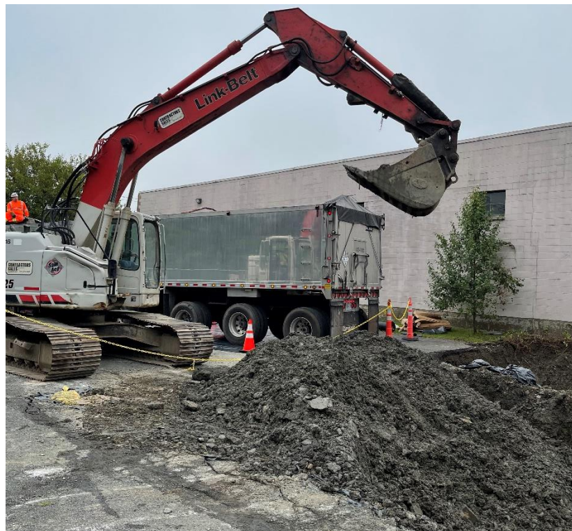
Photograph 22: Loading stockpiled hazardous soil within lined portion of IRM excavation for offsite disposal to Signaterre Environmental, Inc. in Quebec, Canada. View looking southeast. (Photo taken 9/14/21)
