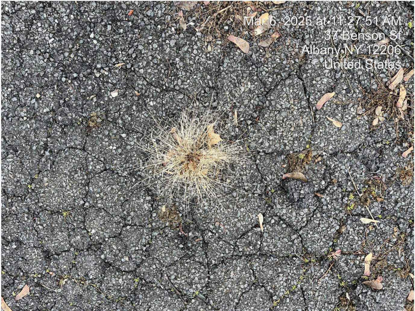
Photo 7 – Broken Pavement area with vegetation
