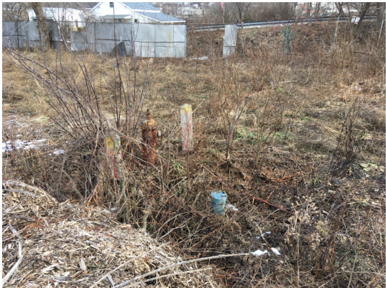
16. Hydrant and Water Valve - Facing East
