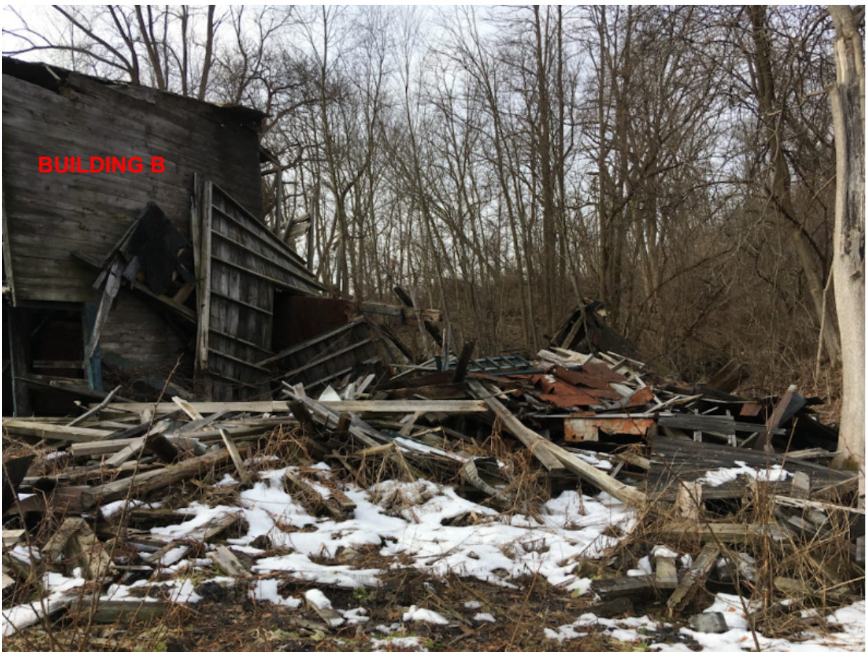
13. Debris Around Building B - Facing West
