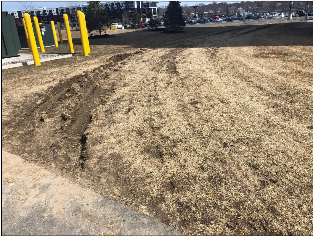
Photo 1. Parcel A – April 3, 2019 Cover Inspection. Minor rutting near Landings Hotel, to be restored.
