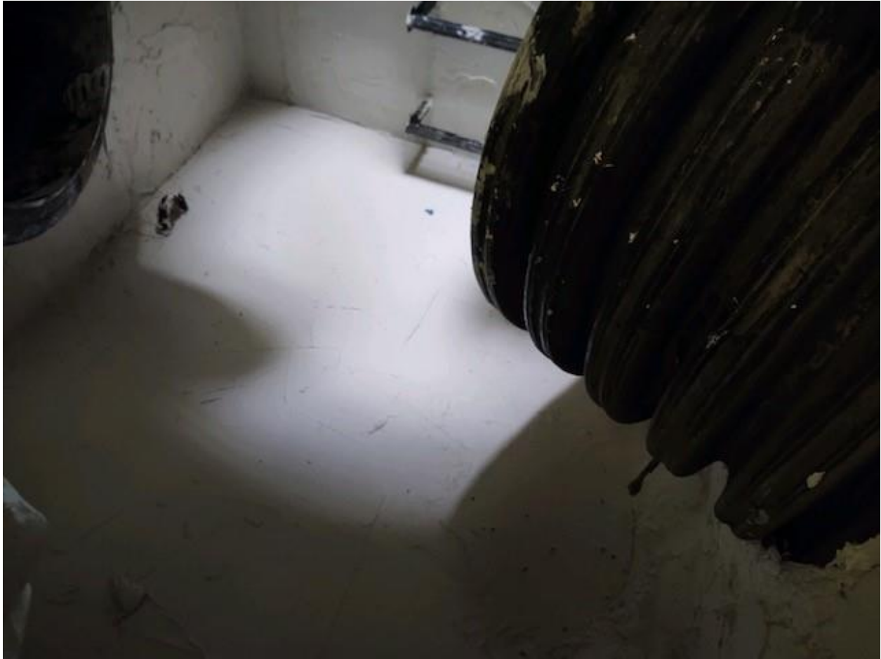
Figure 2: Epoxy seal (DS-1 floor)
