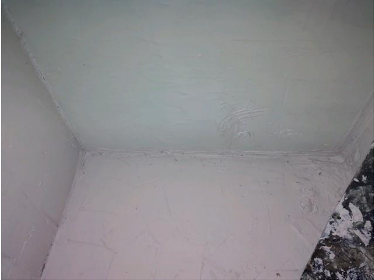
Figure 3: Epoxy Seal (DS-1 floor)
