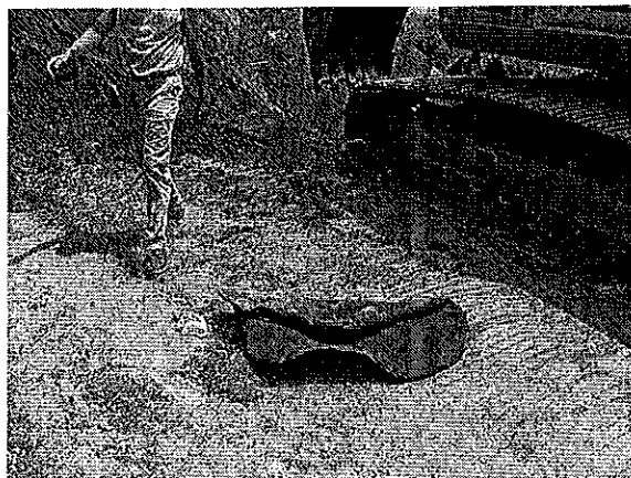
End of UST found in excavation
