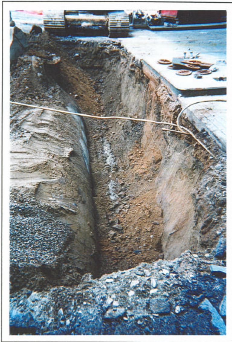
Photograph 8: View to the west of the north wall of the gasoline UST pit
