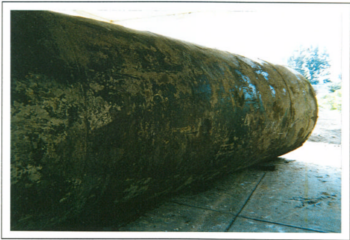
Photograph 6: View of the northern gasoline UST
