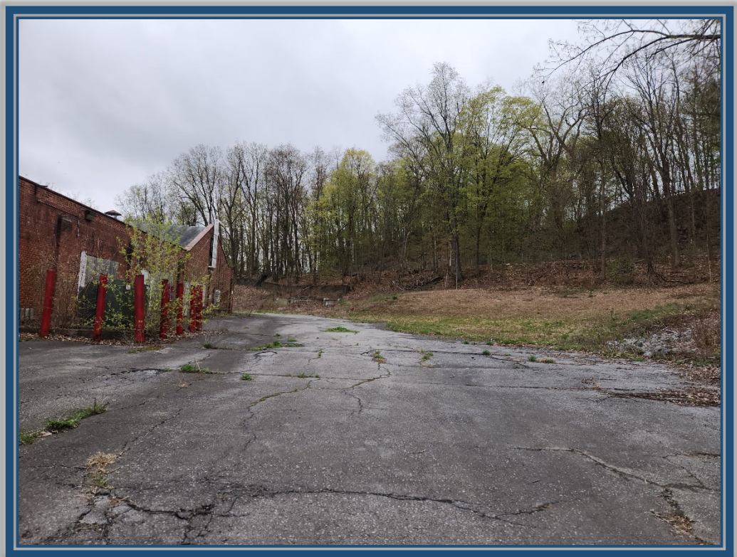
Asphalt surface & soil / Rip Rap cover systems at northwest corner of the Site
