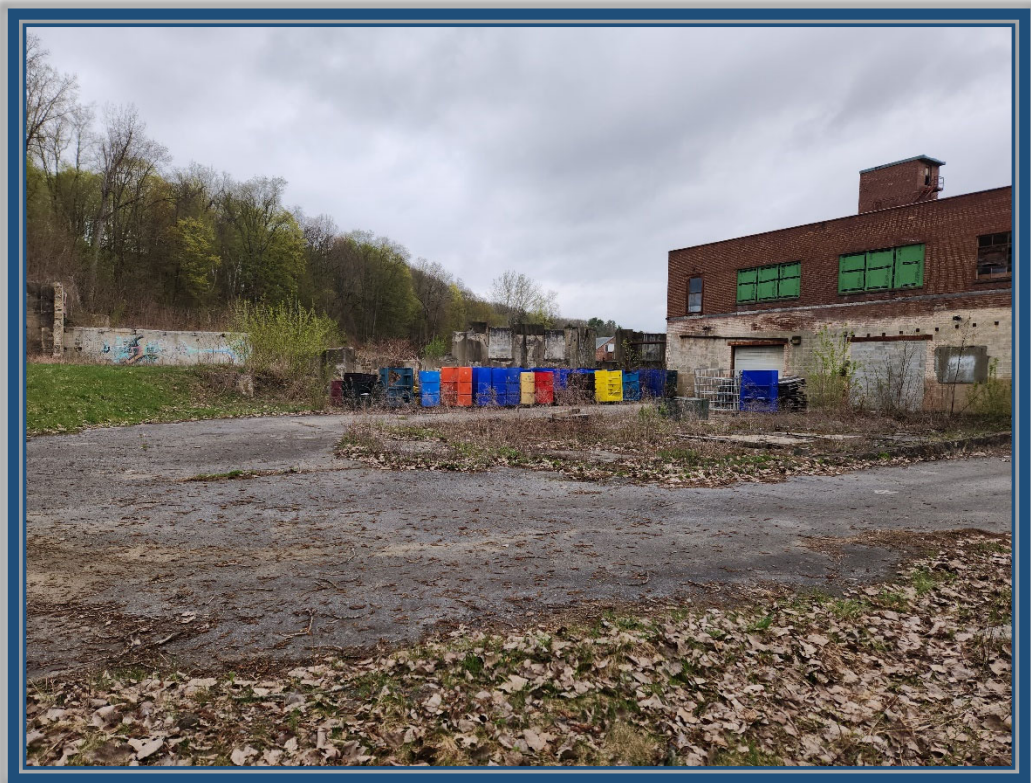
Asphalt & gravel cover systems adjacent to soil cover system southwest of building
