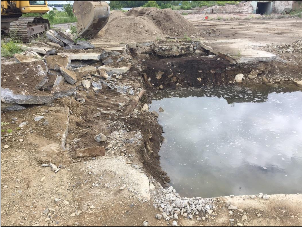
Additional excavation of soils to the north and east of the 20' x 20' excavation area.
