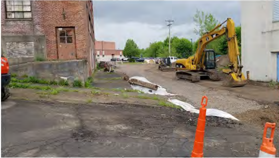
Helen Drive near Avenue B, looking west. Secondary pile of gasoline-contaminated soil and "demarcation barrier" between Helen Drive trench and adjacent Avenue B soils. 2022-05-16 13:21
