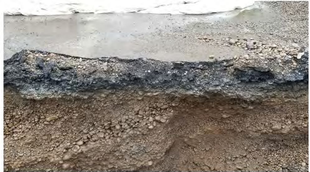
Helen Drive asphalt with discrete layer of gray-stained gasoline-contaminated soils directly beneath. 2022-05-16 13:43
