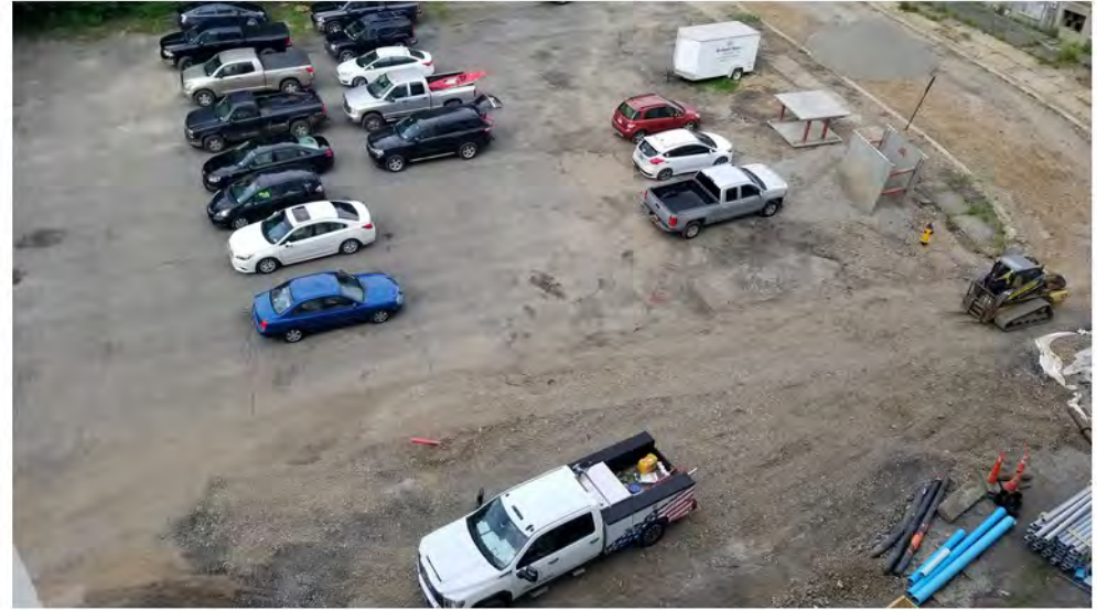
2022-06-01 08:13 42.1159546 N , 75.9518045 W Aerial view of Helen Drive (Work Zone #1), looking south (Avenue B in upper right corner)
