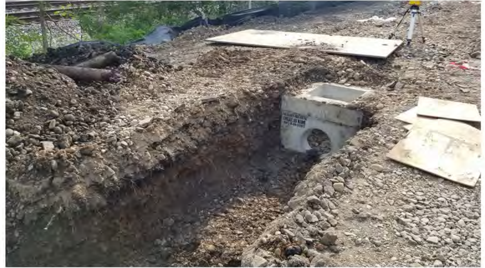
2022-06-01 08:54 42.1281963 N , 75.9533738 W Typical storm catch basin installation along Avenue C
