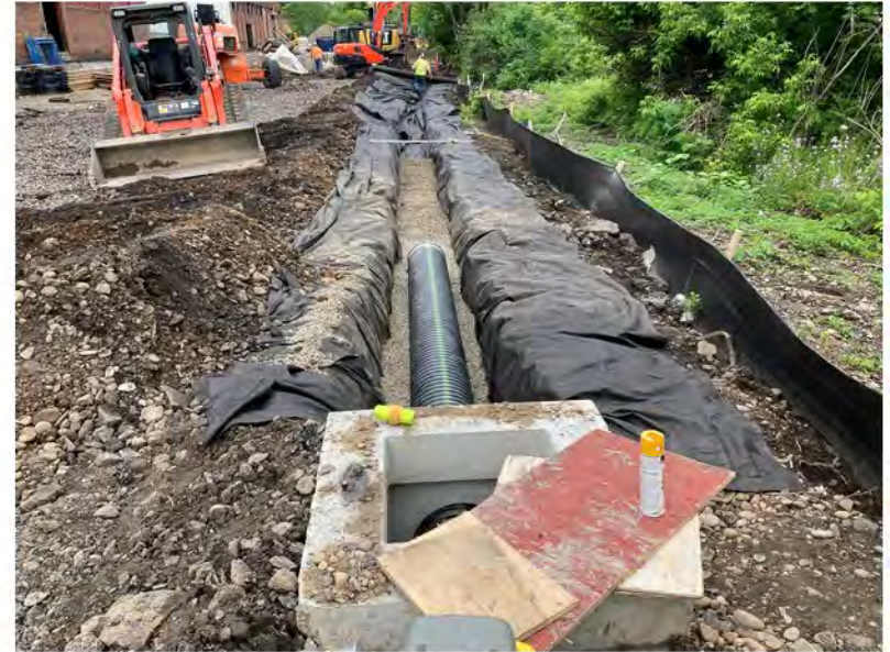
2022-06-02 11:51 42.1152639 N , 75.9527278 W Installation of storm sewer piping, bedding, and filter fabric (not demarcation barrier)
