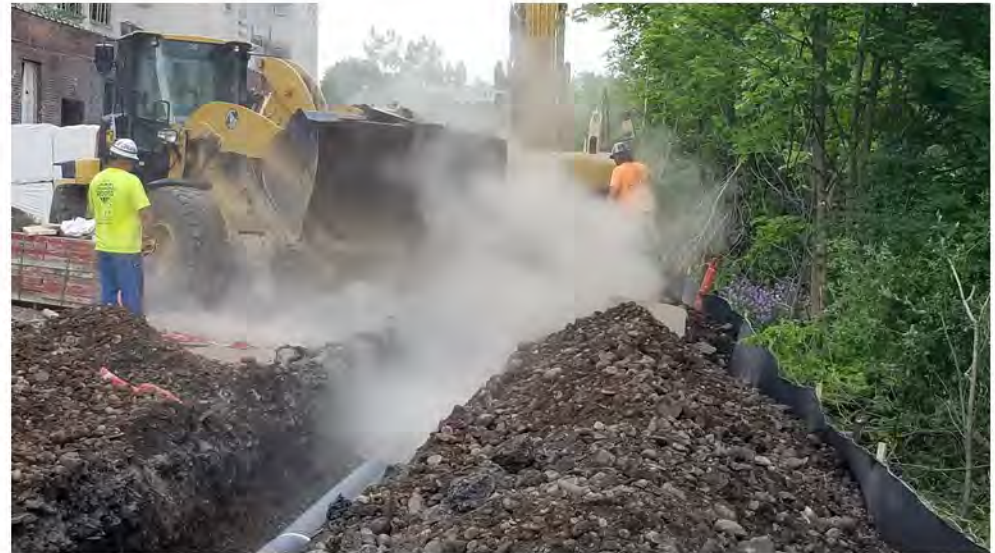
2022-06-01 09:20 42.1157381 N , 75.9508434 W Typical dust created during dumping of clean approved stone bedding material, resulting in some particulate CAMP exceedances
