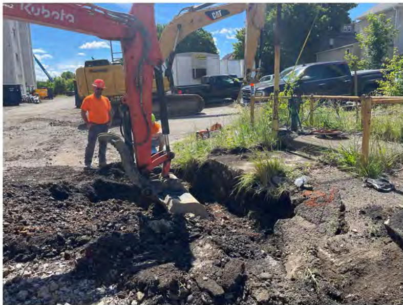
2022-06-10 10:42 42.1154361 N , 75.9517889 W Installation of water line along Helen Drive near corner of Avenue A
