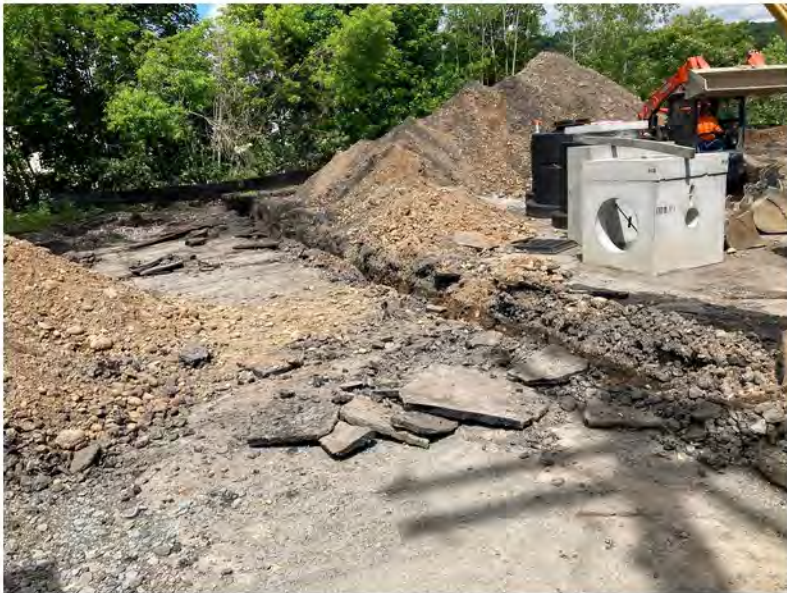
2022-06-09 14:23 42.1159972 N , 75.9533306 W Installation of storm sewer line along the western portion of Avenue C, looking north
