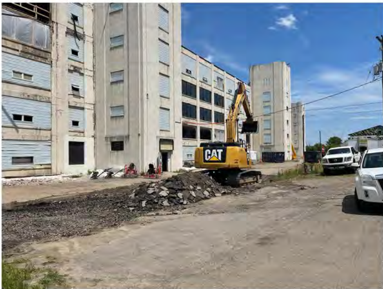
2022-06-06 13:59 42.1153917 N , 75.9521111 W Removal of asphalt along Helen Drive between Avenues A and B
