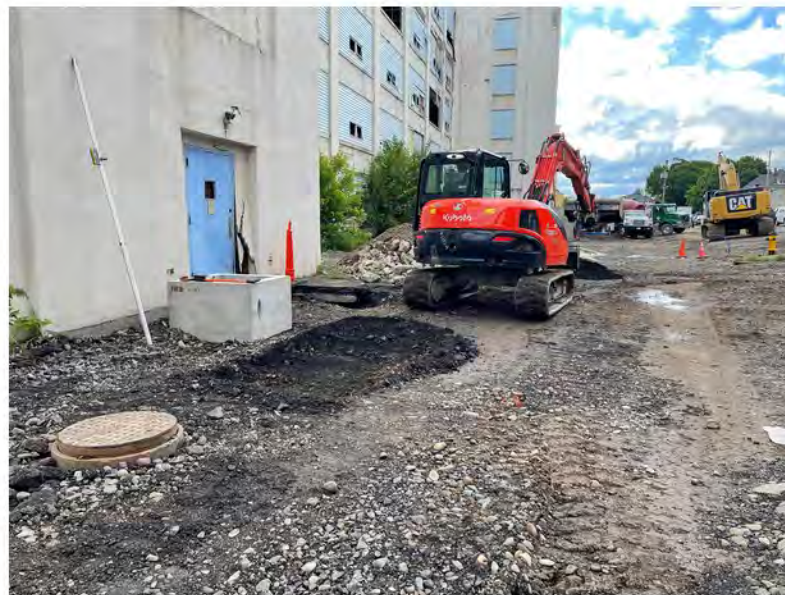
2022-06-08 08:12 42.1157528 N , 75.9530722 W Work Zone #1, installation of storm sewer catch basin near west end of building
