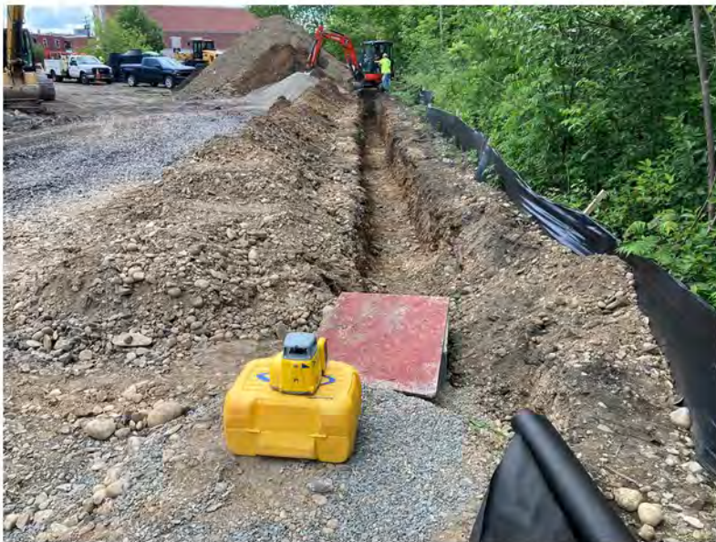
2022-06-08 14:27 42.1161000 N , 75.9526972 W Installation of storm sewer line along Avenue C, looking west
