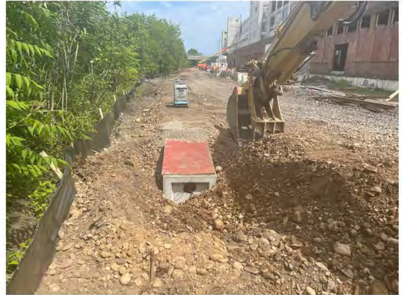
2022-06-06 15:08 42.1160861 N , 75.9535667 W Installation of storm sewer catch basin along Avenue C, looking east
