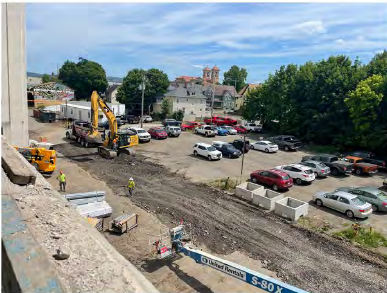
2022-06-06 14:44 42.1156278 N , 75.9522639 W Aerial view of work along Helen Drive between Avenues A and B, looking southeast
