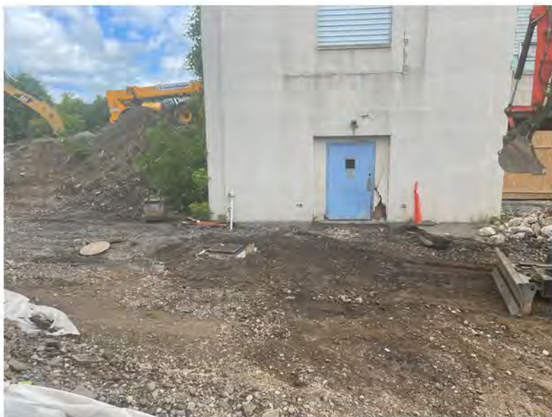
2022-06-08 10:53 42.1156528 N , 75.9529806 W Work Zone #1, installation of storm sewer catch basin near west end of building
