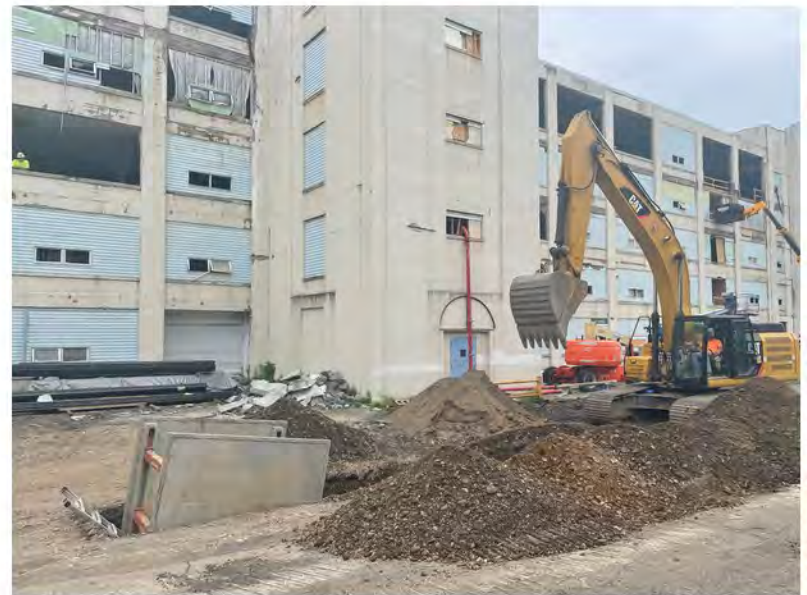
2022-06-07 11:16 42.1151167 N , 75.9526889 W Installation of water line along Helen Drive between Avenues A and B
