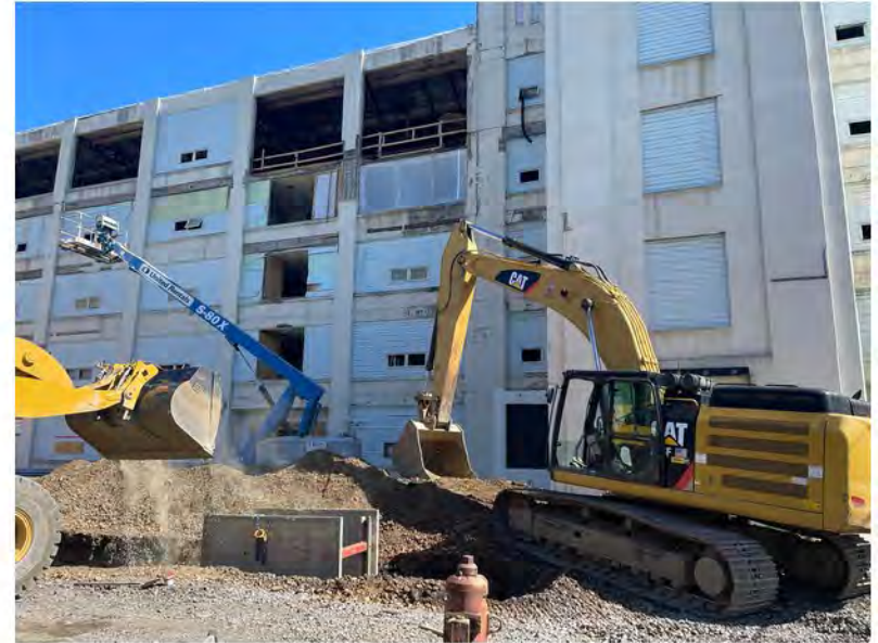
2022-06-10 09:53 42.1153500 N , 75.9518972 W Installation of water line along Helen Drive near corner of Avenue A
