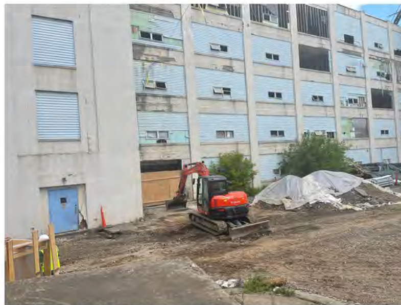
2022-06-08 12:56 42.1155972 N , 75.9528583 W Work Zone #1, installation of storm sewer catch basin near west end of building
