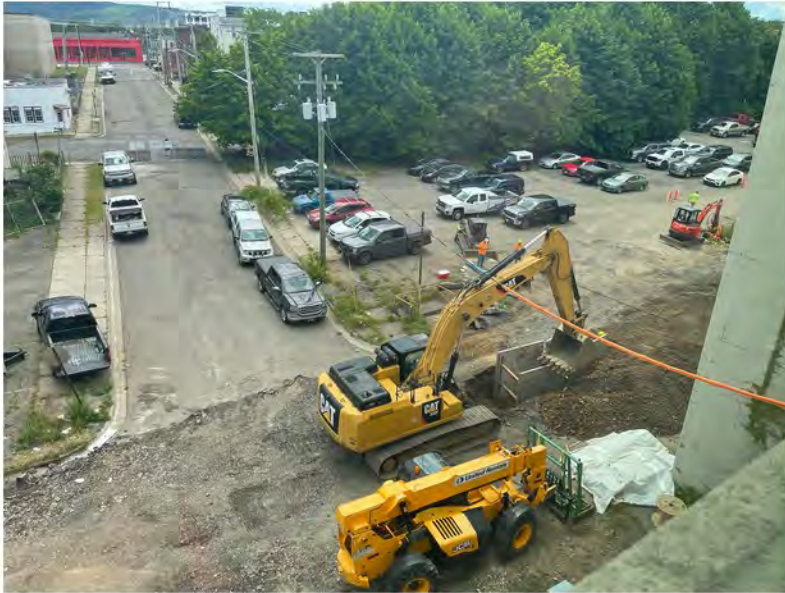
2022-06-10 13:48 42.1155389 N , 75.9517444 W Aerial view of work along Helen Drive, looking south. Avenue A in background.
