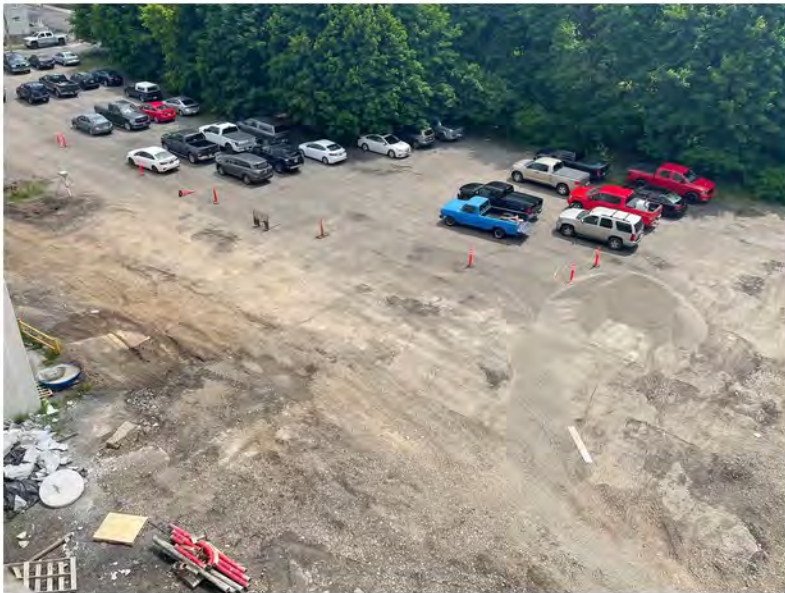
2022-06-10 13:50 42.1157389 N , 75.9526583 W Aerial view of work along Helen Drive between Avenues A and B, looking southeast.
