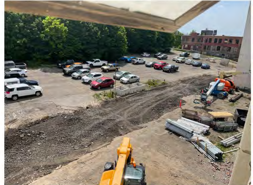
2022-06-06 14:43 42.1154222 N , 75.9518889 W Aerial view of work along Helen Drive between Avenues A and B, looking southwest
