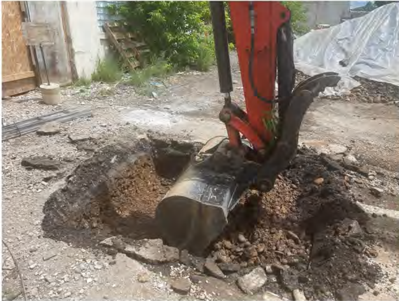
2022-06-08 13:06 42.1156389 N , 75.9529889 W Work Zone #1, installation of storm sewer catch basin near west end of building
