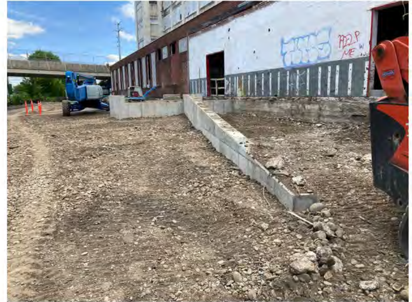
2022-06-08 14:25 42.1156417 N , 75.9512472 W Backfill installed at loading dock along Avenue C, looking east
