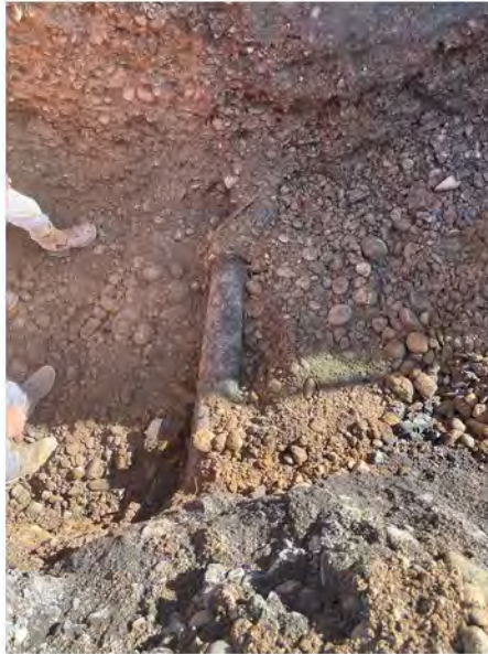
2022-06-10 09:34 42.1154556 N , 75.9518139 W Old water line crossing trench along Helen Drive
