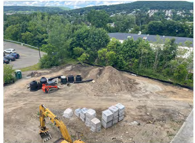
2022-06-10 13:50 42.1158444 N , 75.9529806 W Aerial view of work along western portion of Avenue C, looking northwest.
