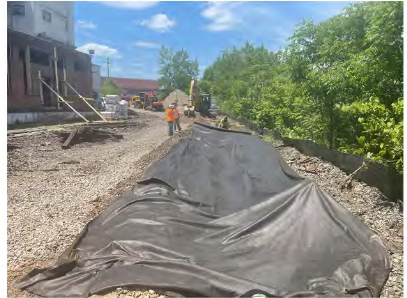
2022-06-06 12:58 42.1160611 N , 75.9523778 W Installation of filter fabric along drainage line in Work Zone #2 (Avenue C), looking west
