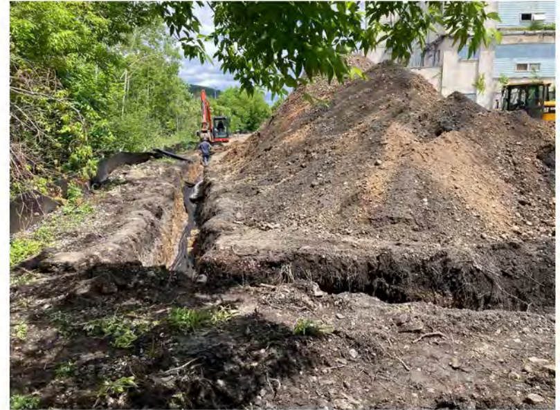
2022-06-09 14:23 42.1164778 N , 75.9533389 W Installation of storm sewer line along the western portion of Avenue C, looking east
