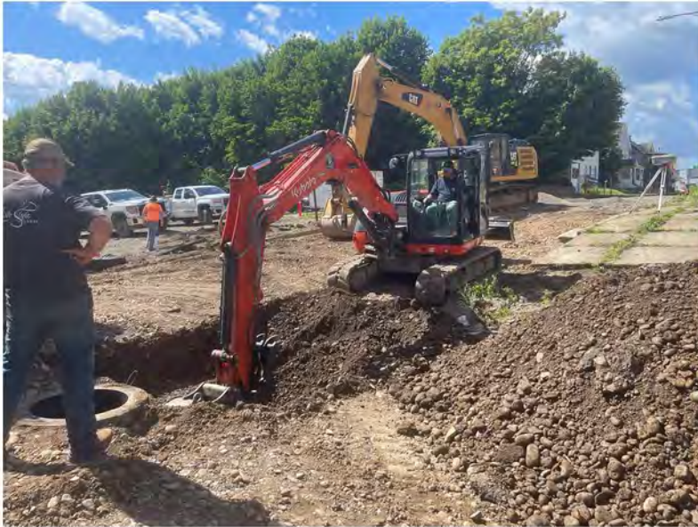
2022-06-17 10:19 42.1158167 N , 75.9529639 W Storm sewer excavation at intesection of Helen Drive and Avenue B, looking southeast
