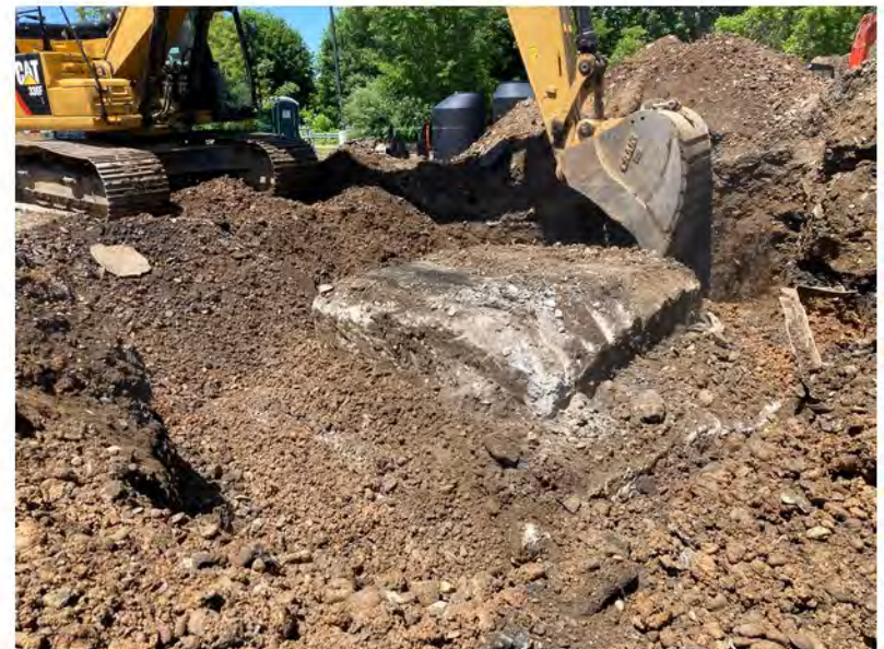
2022-06-13 13:21 42.1158472 N , 75.9530861 W Large concrete block in western end of Work Zone #2 (Avenue C)
