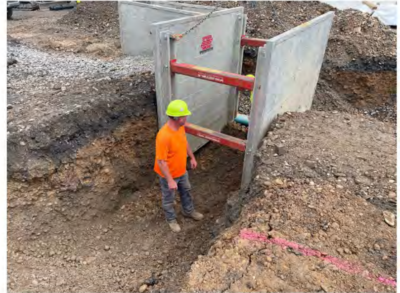
2022-06-13 10:07 42.1153222 N , 75.9518194 W Helen Drive storm sewer excavations near west end of building, looking north
