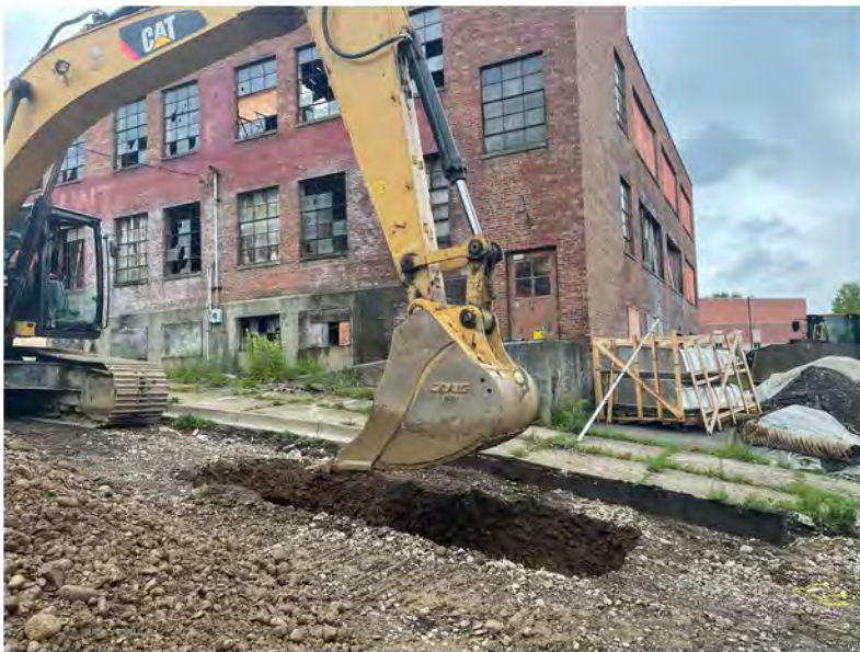
2022-06-16 08:49 42.1156500 N , 75.9528500 W Storm sewer excavation at intesection of Helen Drive and Avenue B, looking west
