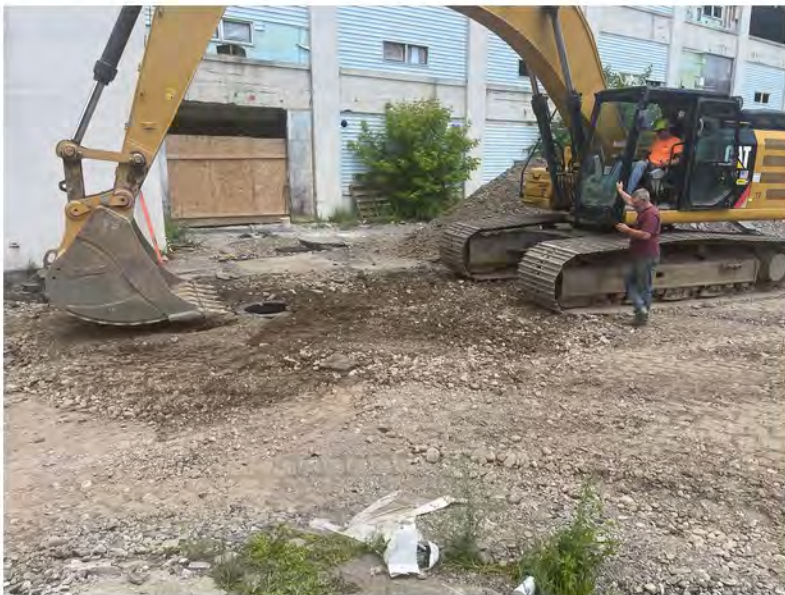
2022-06-15 13:20 42.1157000 N , 75.9529278 W Storm sewer catch basin installed along Helen Drive, near Avenue B
