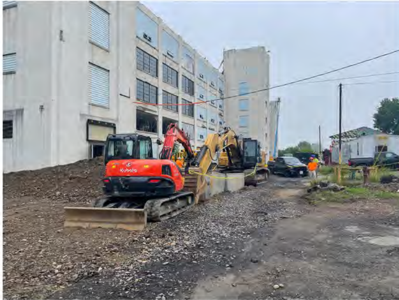
2022-06-13 07:51 42.1148917 N , 75.9519194 W Work Zone #1 (Helen Drive), storm sewer excavations near west end of building, looking east
