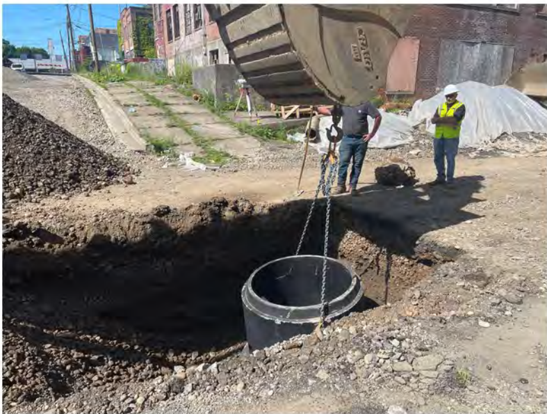
2022-06-15 10:09 42.1153444 N , 75.9529278 W Installation of storm sewer catch basin at intersection of Avenue B and Helen Drive, looking south
