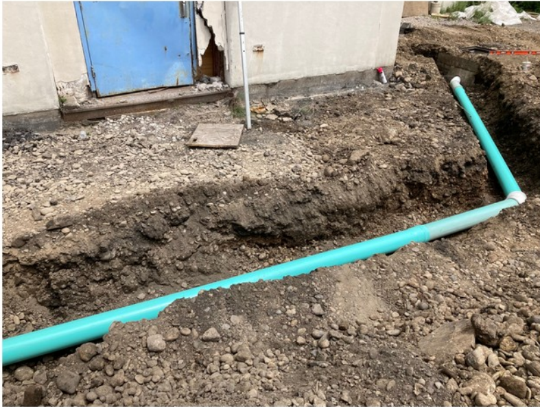
2022-06-22 12:59 42.1157806 N , 75.9529417 W Work Zone #1 (Helen Drive) storm sewer installation at west end of building
