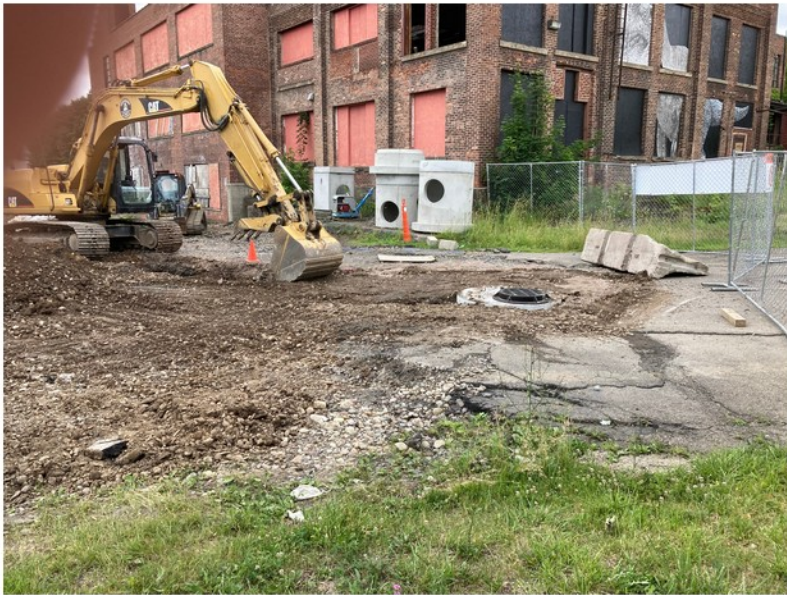
2022-06-23 12:05 42.1158472 N , 75.9534917 W Storm sewer installation at west end of site, looking southeast
