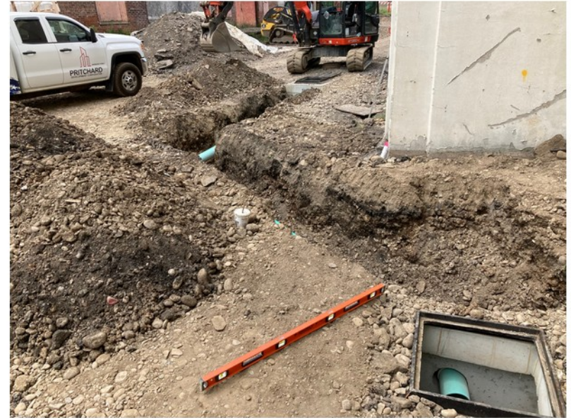
2022-06-22 12:59 42.1157583 N , 75.9528278 W Work Zone #1 (Helen Drive) storm sewer installation at west end of building
