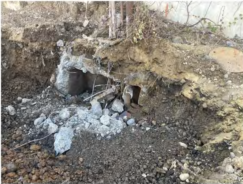
2022-07-01 10:48 42.1155028 N , 75.9533222 W Vault with asbestos-clad pipe at west end of building. Work stopped.
