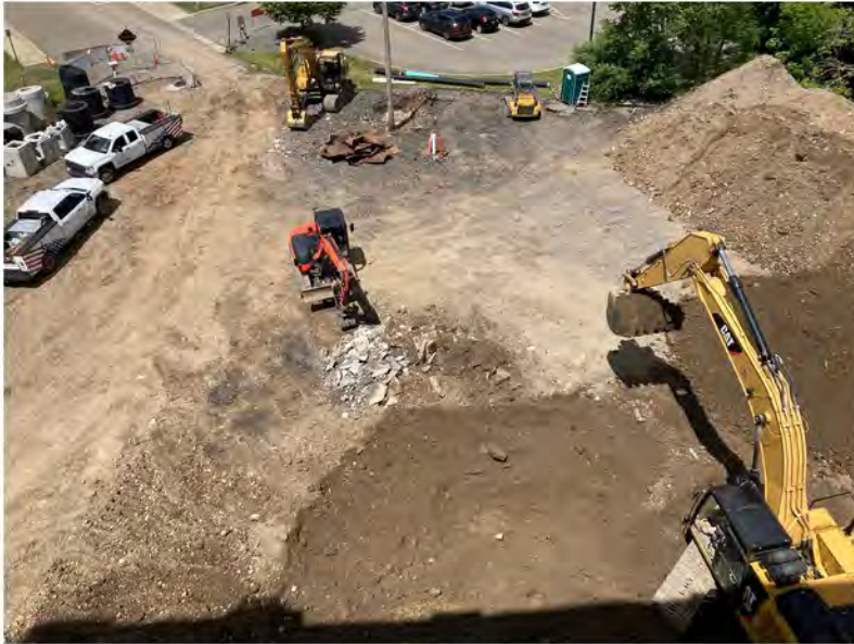
2022-06-28 11:53 42.1158750 N , 75.9529722 W Aerial view of ramp removal at west end of site, looking west
