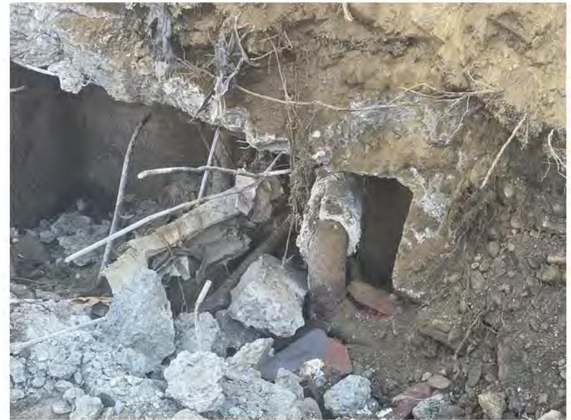
2022-07-01 10:48 42.1157194 N , 75.9532000 W Vault with asbestos-clad pipe at west end of building. Work stopped.
