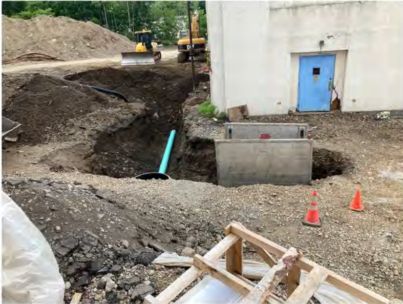
2022-07-06 15:55 42.1156278 N , 75.9529722 W Sewer work on Helen Drive (Work Zone #1) near the western end of the building
