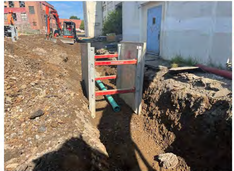
2022-07-11 09:44 42.1151861 N , 75.9524917 W Installation of sewer line along Helen Drive near Avenue A, looking west
