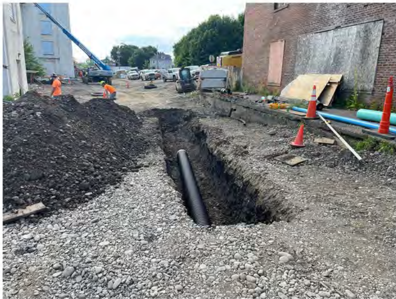
2022-07-12 09:06 42.1158722 N , 75.9532167 W Installation of storm sewer line along Helen Drive near western property border, looking east
