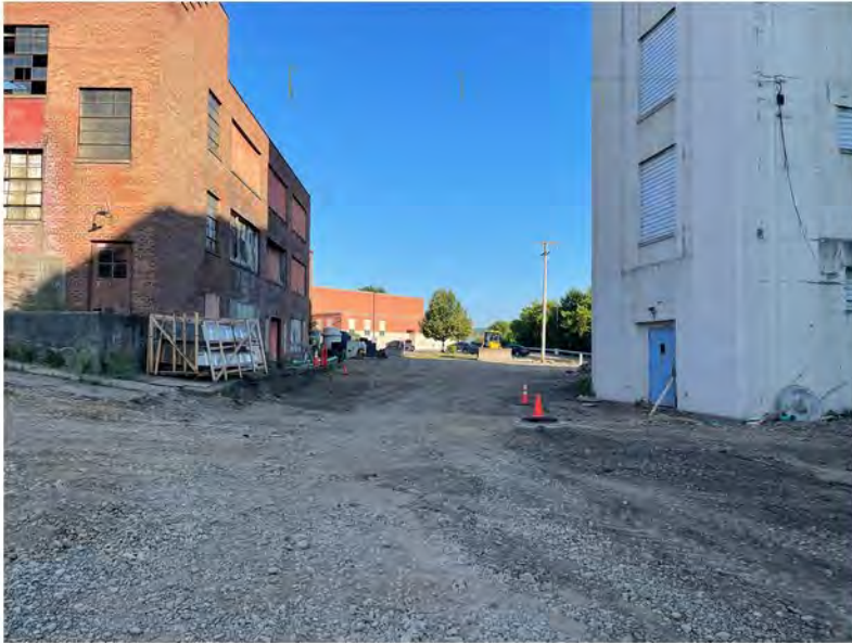
2022-07-11 07:42 42.1151194 N , 75.9531111 W West end of Helen Drive near Avenue B (Work Zone #1), looking west
