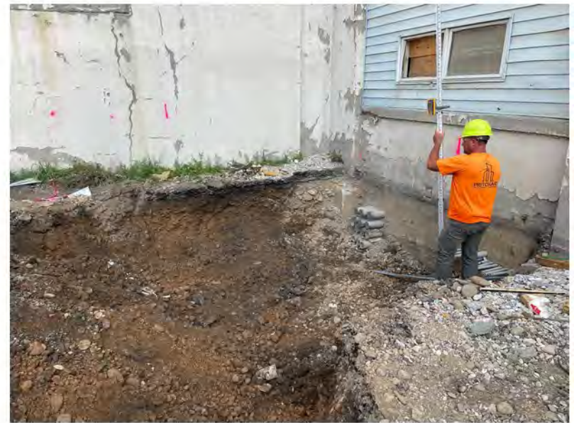
2022-07-12 09:15 42.1156306 N , 75.9521639 W Excavation for electric vault along southern side of the building, looking west
