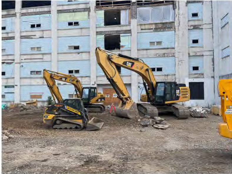
2022-07-12 07:26 42.1154056 N , 75.9519056 W Backfilling of sewer line trenches along Helen Drive near Avenue A
