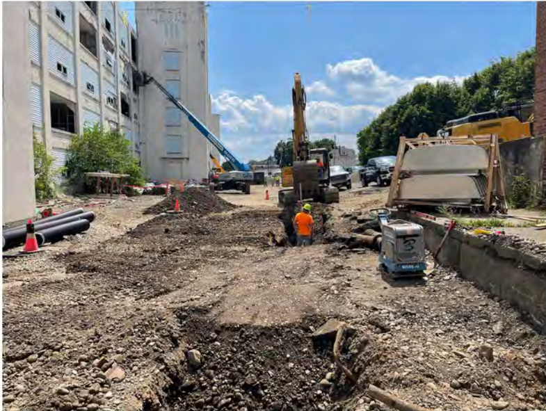
2022-07-12 11:32 42.1157500 N , 75.9531167 W Installation of sewer line along Helen Drive near Avenue B, looking east
