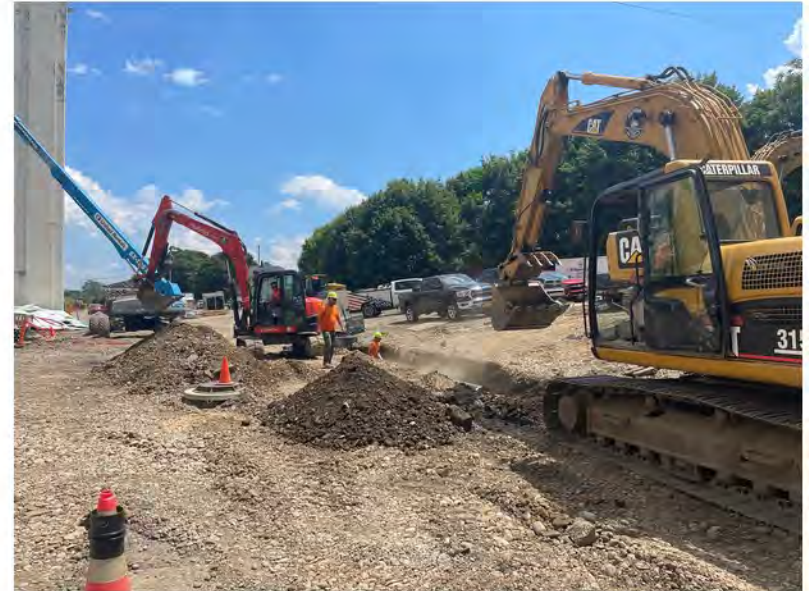
2022-07-12 13:49 42.1157083 N , 75.9530333 W Installation of sewer line along Helen Drive near Avenue B, looking southeast
