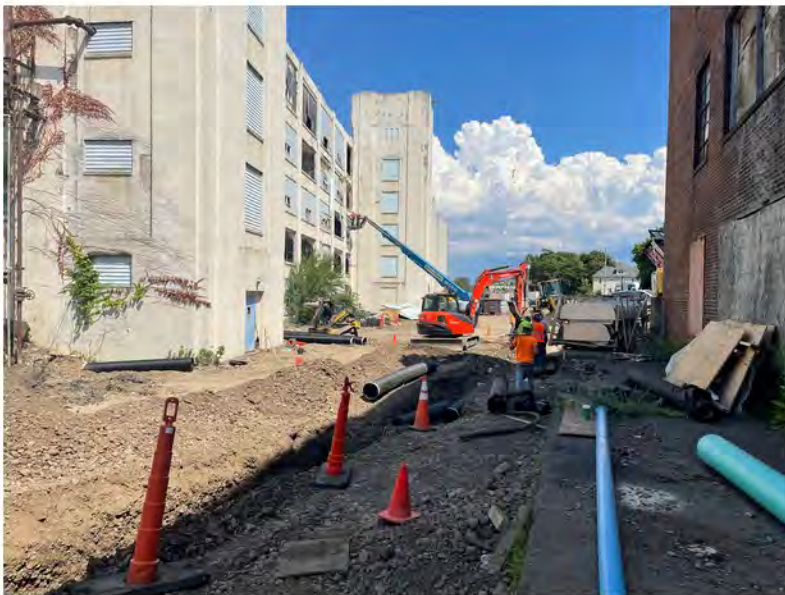
2022-07-12 15:14 42.1161722 N , 75.9532389 W Installation of storm sewer line along Helen Drive near western property border, looking east
