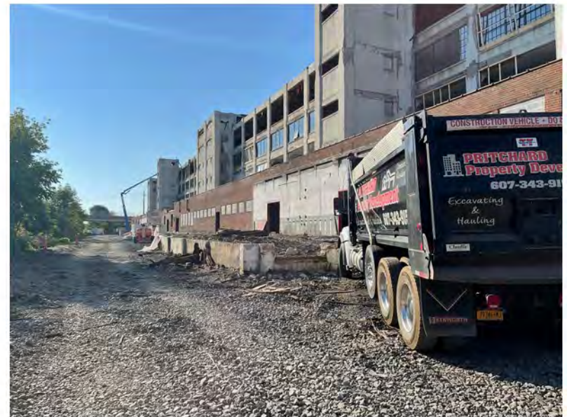
2022-07-11 08:09 42.1158722 N , 75.9523250 W Avenue C (north side of building), preparing for material load-out
