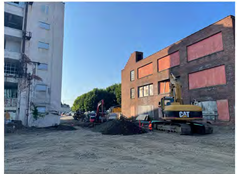
2022-07-13 08:03 42.1160611 N , 75.9531778 W Installation of storm sewer line along Helen Drive near western property border, looking southeast
