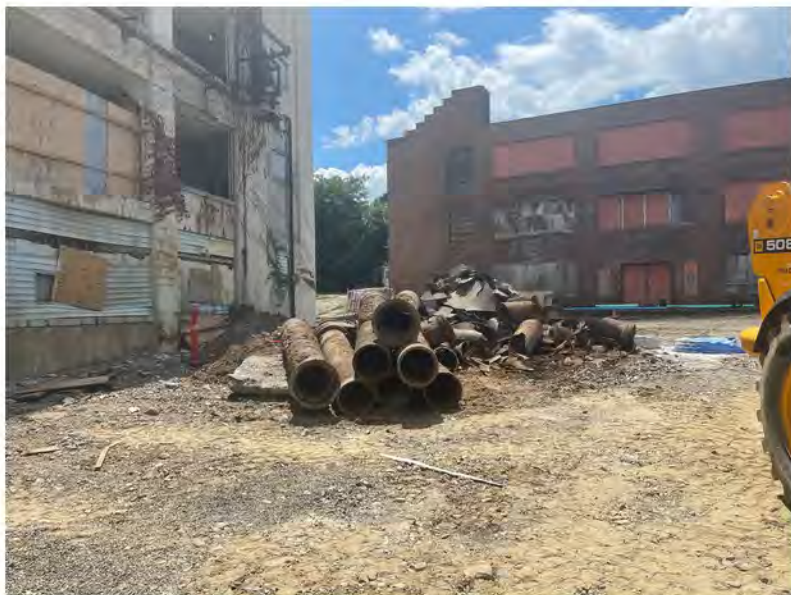
2022-07-21 13:01 42.1160056 N , 75.9529639 W Sewer lines (excavated from Helen Drive) staged on west end of building
