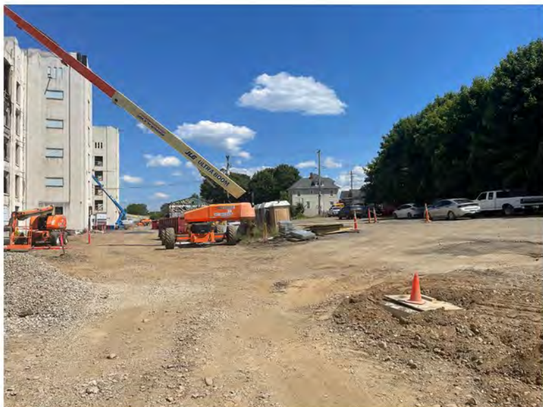
2022-07-22 15:06 42.1156111 N , 75.9524306 W Western portion of site, looking east down Helen Drive (Avenue B to right)
