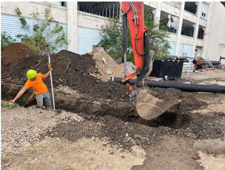
2022-07-28 09:52 42.1157139 N , 75.9531639 W Trenching for sewer lines from main building to Helen Drive catch basins
