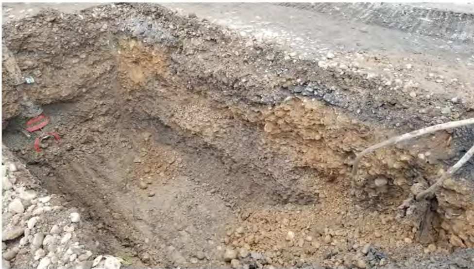
2022-07-25 13:20 42.1154510 N , 75.9516877 W Trench for new water line at intersection of Helen Drive and Aveune A
