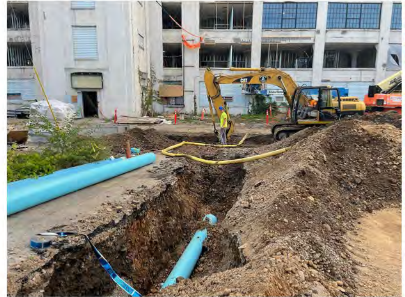
2022-07-26 07:33 42.1152389 N , 75.9517056 W Installation of water line along Avenue A (outside of BCP area)
