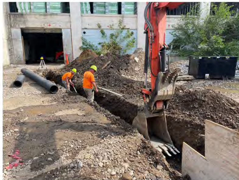
2022-07-28 10:05 42.1148694 N , 75.9527361 W Trenching for sewer lines from main building to Helen Drive catch basins
