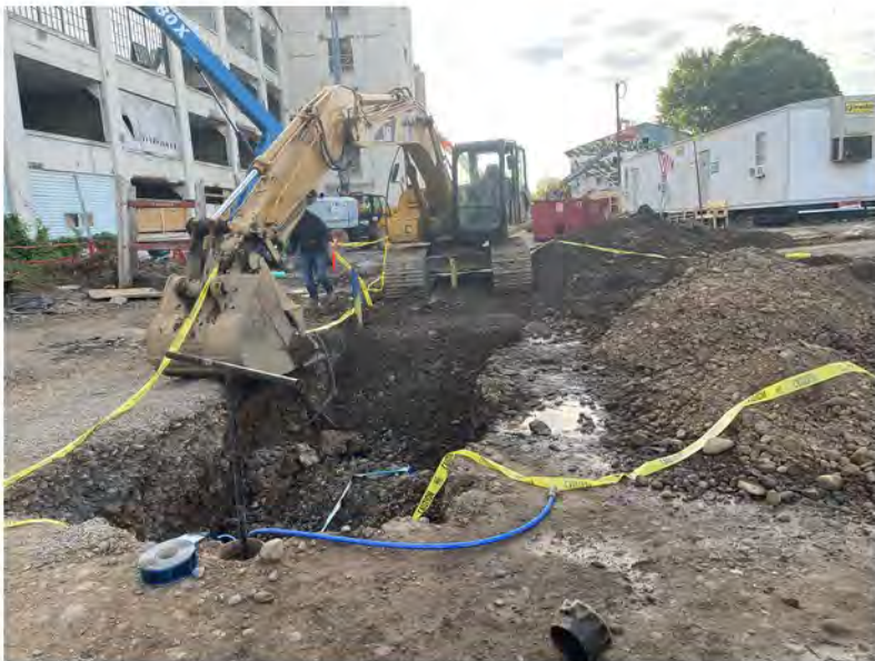
2022-07-27 07:32 42.1147500 N , 75.9517222 W Backfilling trench at intersection of Helen Drive and Avenue A, looking east
