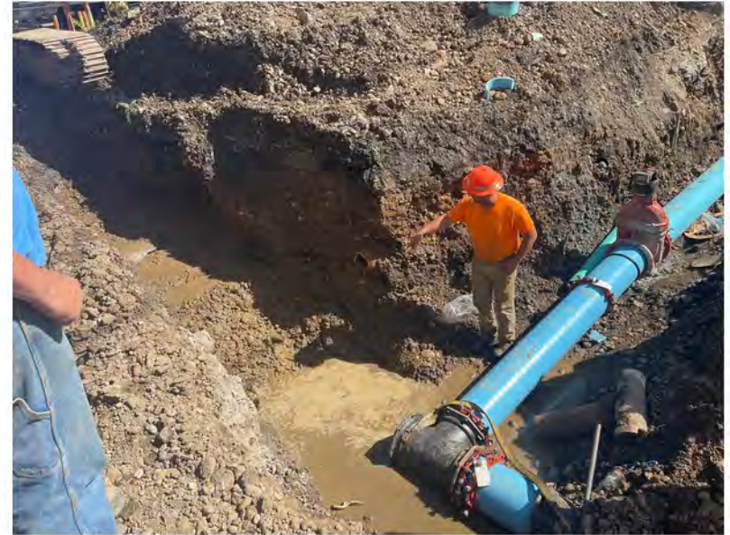
2022-07-26 16:08 42.1153833 N , 75.9516611 W Installation of new water pipe at intersection of Helen Drive and Aveune A
