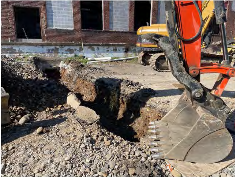
2022-07-29 09:22 42.1156389 N , 75.9506750 W Trenching for sewer lines from annex to Avenue C catch basins
