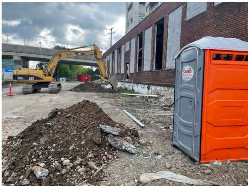
2022-07-28 09:57 42.1156111 N , 75.9508750 W Trenching for sewer lines from annex to Avenue C catch basins
