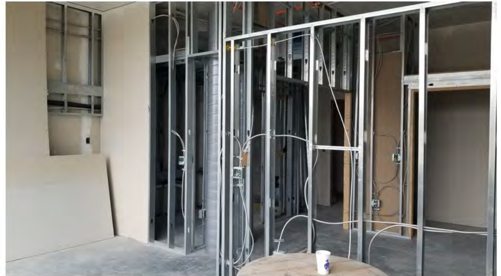
2022-07-25 08:43 42.1150422 N , 75.9512074 W Status of interior renovations on 3rd Floor (FOR INFO ONLY)
