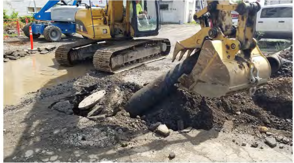
2022-07-25 11:09 42.1153449 N , 75.9517642 W Removal of sewer line at intersection of Helen Drive and Aveune A
