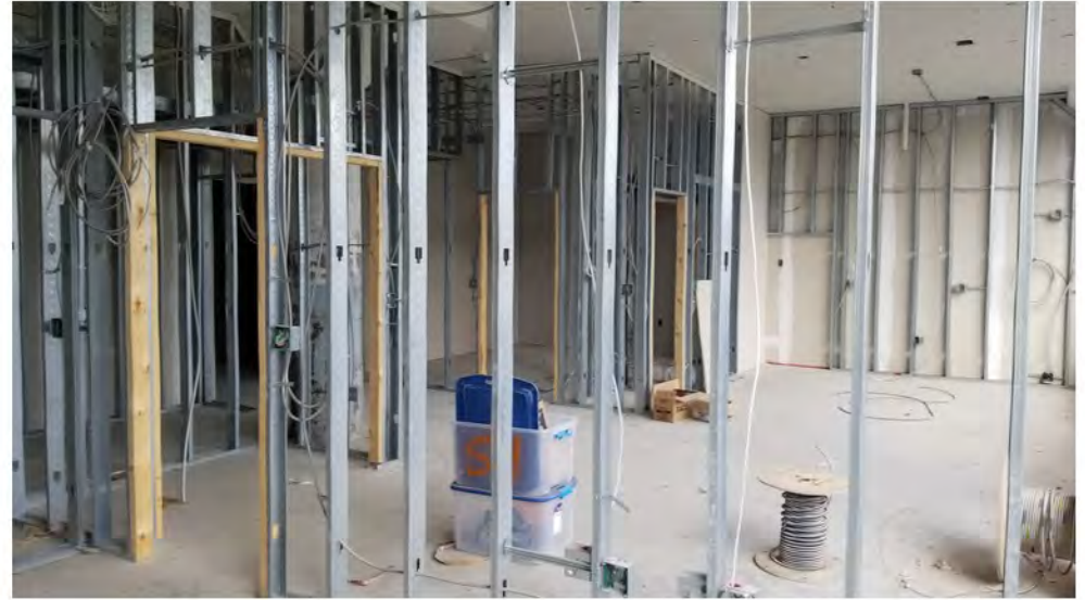
2022-07-25 08:45 42.1165224 N , 75.9505762 W Status of interior renovations on 2nd Floor (FOR INFO ONLY)
