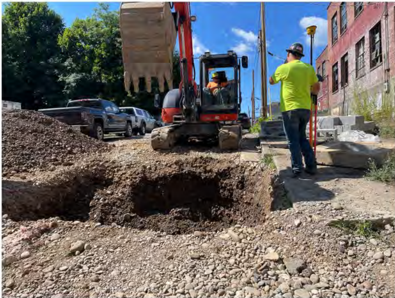
2022-07-29 10:45 42.1156972 N , 75.9529028 W Excavating old catch basin on Avenue B at Helen Drive
