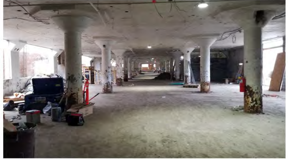
2022-07-25 08:51 42.1151455 N , 75.9515079 W Status of interior renovations on Ground/1st Floor (FOR INFO ONLY)
