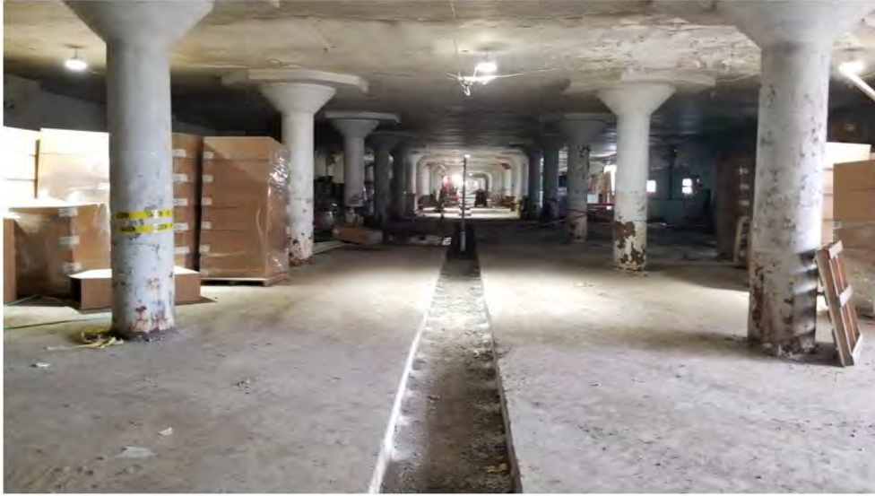
2022-07-25 08:50 42.1161638 N , 75.9537628 W Status of interior renovations on Ground/1st Floor (FOR INFO ONLY)
