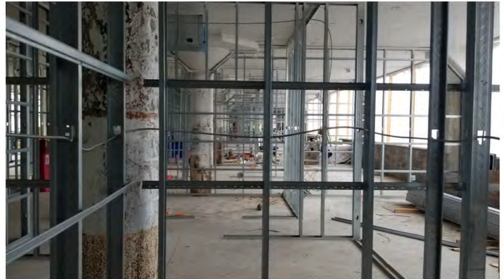
2022-07-25 08:47 42.1150336 N , 75.9516115 W Status of interior renovations on 2nd Floor (FOR INFO ONLY)
