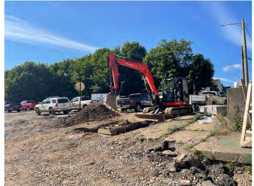
2022-07-29 09:30 42.1157083 N , 75.9529806 W Excavating old catch basin on Avenue B at Helen Drive
