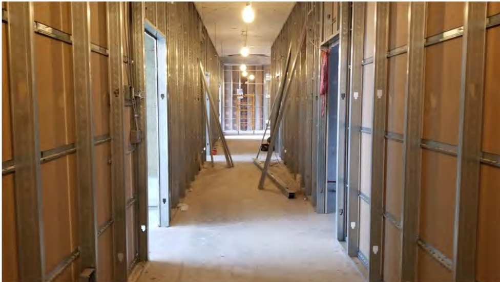
2022-07-25 08:41 42.1155942 N , 75.9516076 W Status of interior renovations on 3rd Floor (FOR INFO ONLY)
