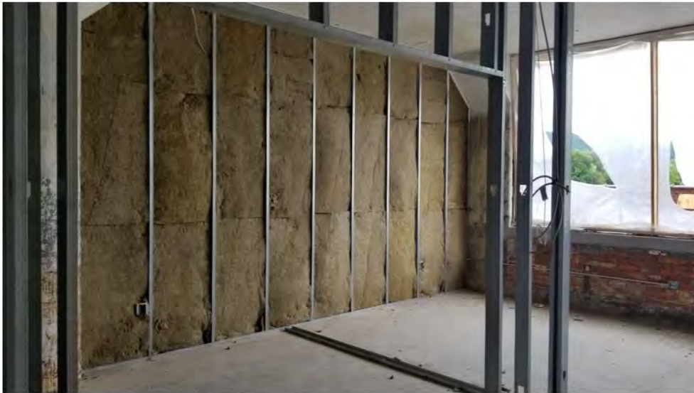
2022-07-25 08:47 42.1157285 N , 75.9518214 W Status of interior renovations on 2nd Floor (FOR INFO ONLY)
