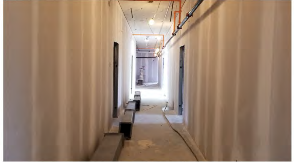
2022-07-25 08:40 42.1151687 N , 75.9531322 W Status of interior renovations on 4th Floor (FOR INFO ONLY)
