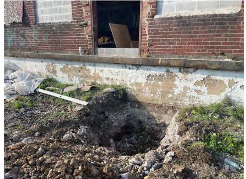
2022-07-28 08:18 42.1156056 N , 75.9507528 W Beginning sewer line extension from annex to Avenue C catch basins
