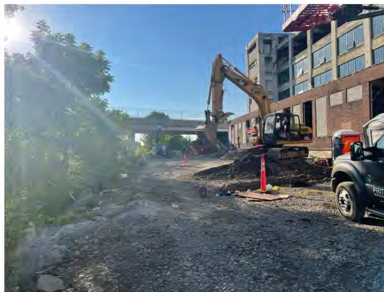
2022-07-29 07:53 42.1157583 N , 75.9511333 W Trenching for sewer lines from annex to Avenue C catch basins, looking east
