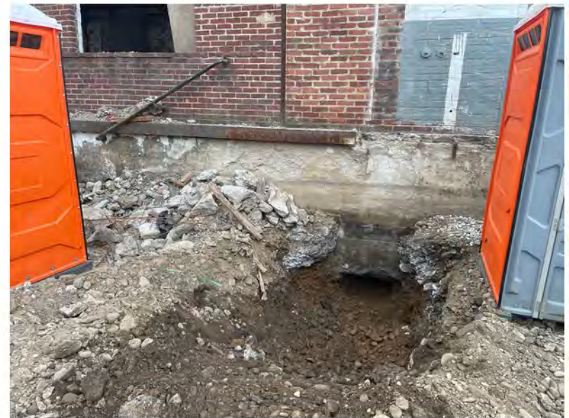
2022-07-28 09:57 42.1155889 N , 75.9508528 W Beginning sewer line extension from annex to Avenue C catch basins
