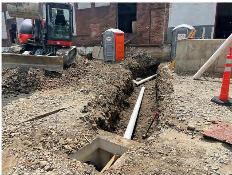
2022-07-28 12:55 42.1157500 N , 75.9509583 W Trenching for sewer lines from annex to Avenue C catch basins
