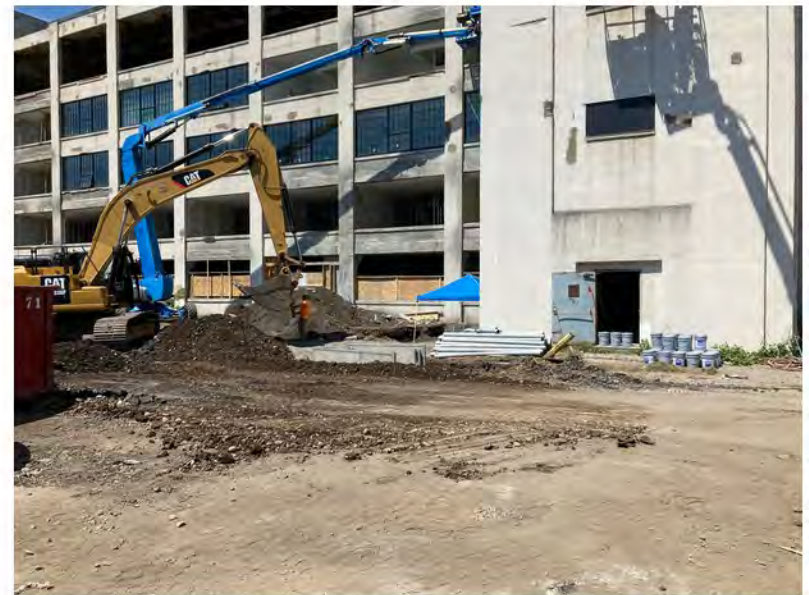
2022-08-03 14:25 42.1151806 N , 75.9511417 W Excavation along Helen Drive, near the eastern end of the building
