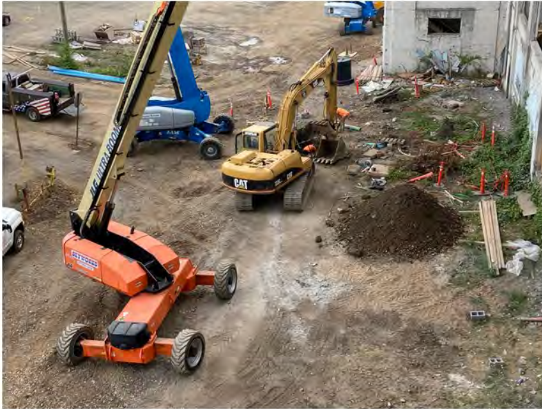
2022-08-04 13:22 42.1154139 N , 75.9514167 W Aerial view of excavation on Helen Drive near Avenue A
