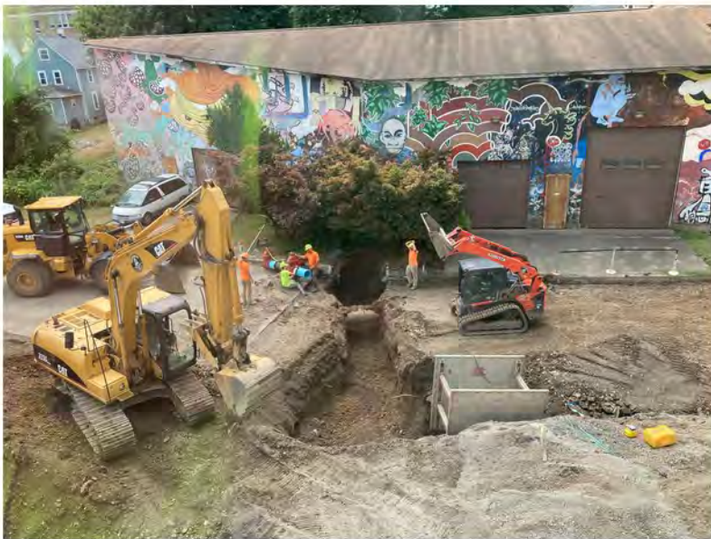
2022-08-05 13:16 42.1155778 N , 75.9491806 W Aerial view of excavations on Helen Drive near eastern end of building, looking south
