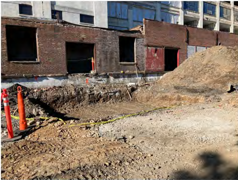
2022-08-12 08:40 42.1159333 N , 75.9514833 W Work Zone #2 (northern excavations), cooling tower foundation excavation along Avenue C
