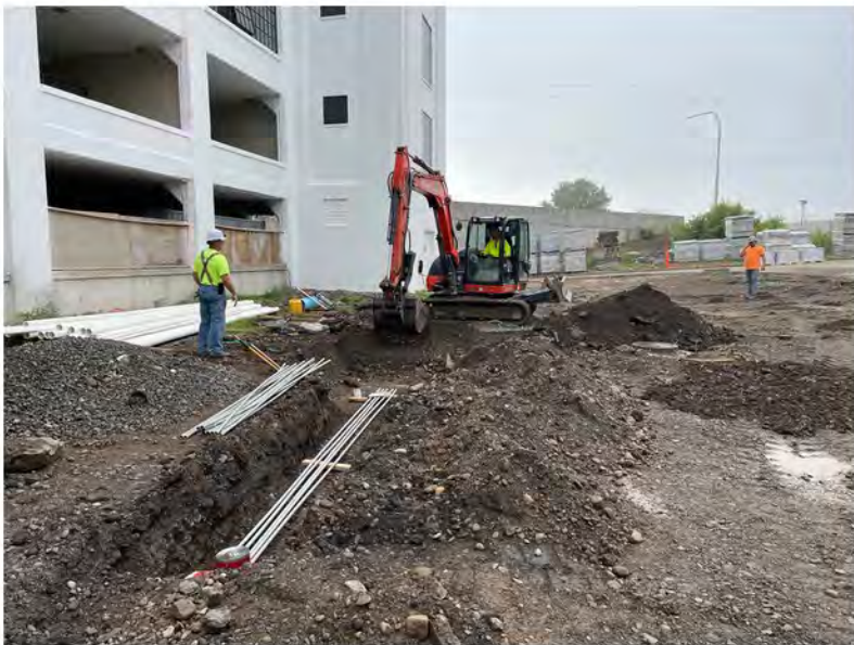
2022-08-19 08:35 42.1152583 N , 75.9508889 W Excavations for electric conduit along Helen Drive, near east end of building
