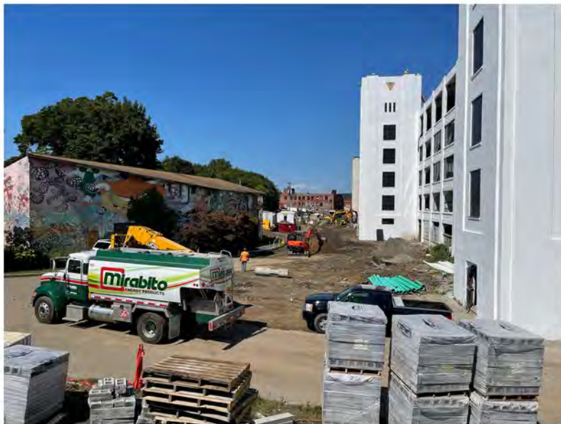
2022-08-19 11:22 42.1151389 N , 75.9502806 W Excavation and grading/leveling activities along Helen Drive, looking west from Lester Ave
