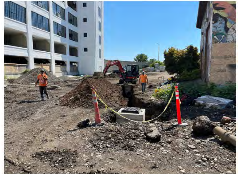
2022-08-19 11:17 42.1152889 N , 75.9511111 W Storm sewer excavation along Helen Drive near Avenue A, looking east
